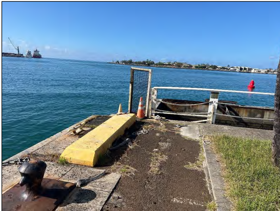
Figure 50. Photo off the west end of Pier 7, notice the concrete docking block and metal cleat, view west
