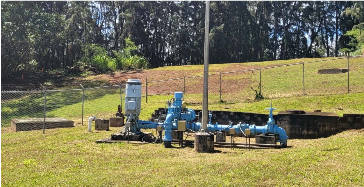
Figure 2-6: Example of Production Well
