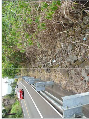
Figure 40. SHIP Site 30187 Feature C, top surface of the lower retaining wall, view to the southeast.
