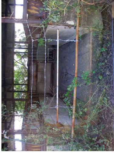
Figure 122. S1HP Site 25507 Feature A, former entryway in the northern side to the western portion of the building, view to the southeast.
