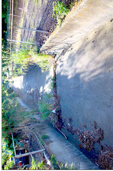
Figure 6. "Area 2" in our survey is a section of concrete-lined drainage channel at Melia Street.
