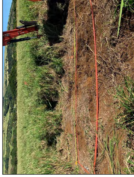
Figure 56. Photograph of TT-3 marked out with flagging tape prior to excavation; view to north
