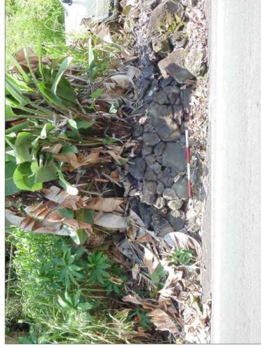
Figure 43. SHP Site 30187 Feature D, section of retaining wall at the southeastern end of abandoned road segment, view to the northeast.
