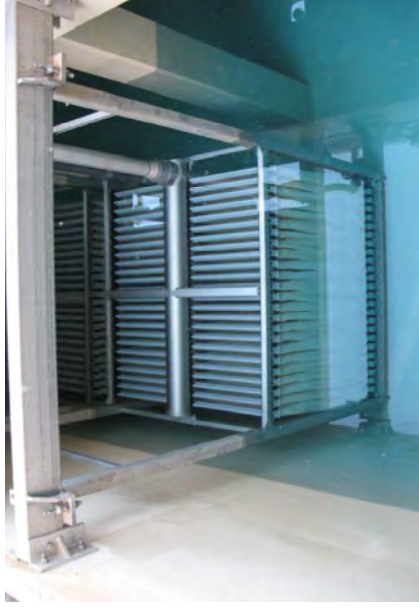
Figure 5-9. Membrane Cassettes at Johns Creek Environmental Campus Fulton County, Georgia
