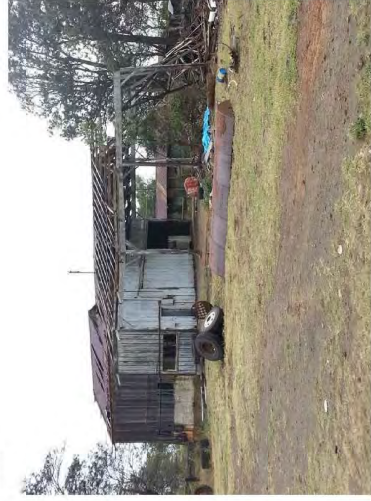
Figure 144. SHEP Site 29507 Feature D, door in north end of the west wall of the main structure, view to the southwest.
