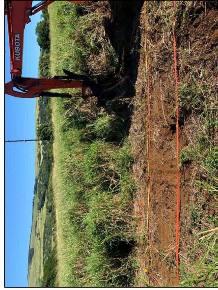
Figure 60. Photograph of TT-4 marked out with flagging tape prior to excavation, view to north
