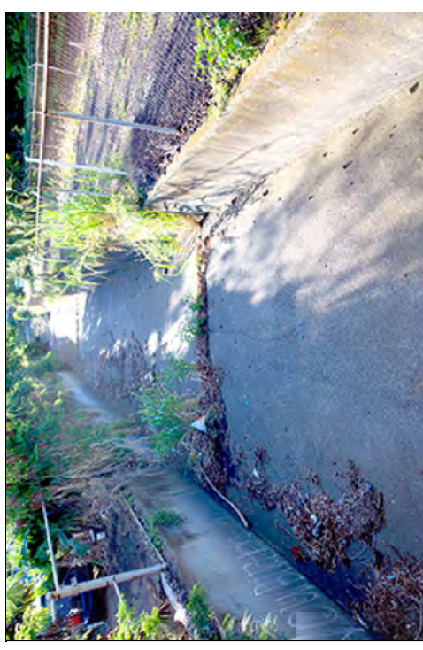
Figure 6. "Area 2" in our survey is a section of concrete-lined drainage channel at Melia Street.
