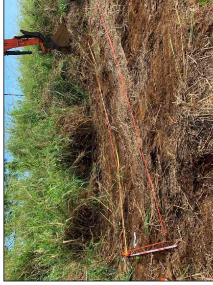
Figure 48. Photograph of TT-1 marked out with flagging tape prior to excavation; view to east
