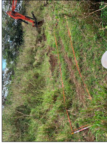
Figure 68. Photograph of TT-6 marked out with flagging tape prior to excavation, view to southeast
