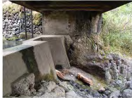
Sluice gate beneath the bridge Courtesy of NOEI
