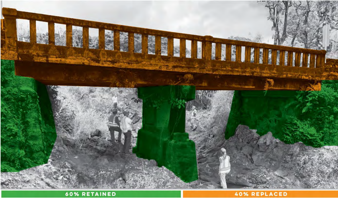
Figure 4: Ulaino Stream Bridge, Overview of Effects and Rendering of the Proposed Action
