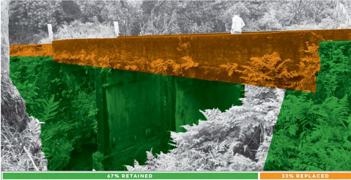
Figure 5: Mokulehua Stream Bridge, Overview of Effects and Rendering of the Proposed Action
