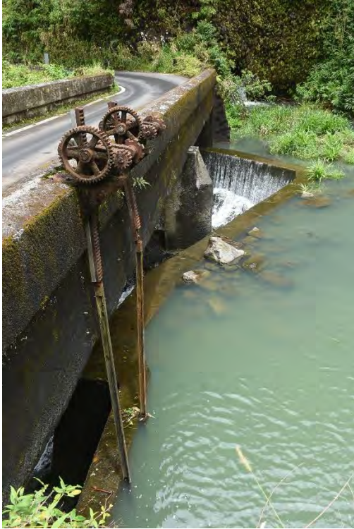
Fig. 19. Kopiliula Stream bridge, 1280 ft., looking east. Note integration of bridge with diversion.
