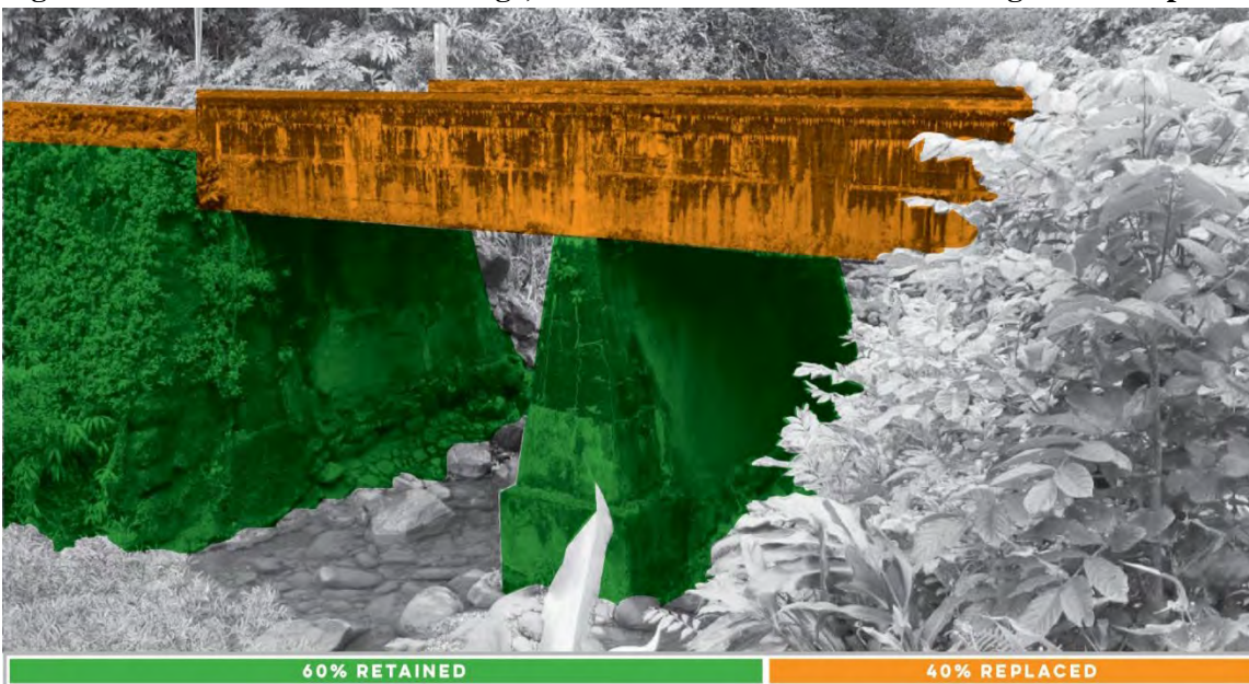
Figure 3: Puohokamoā Stream Bridge, Overview of Effects and Rendering of the Proposed Action
