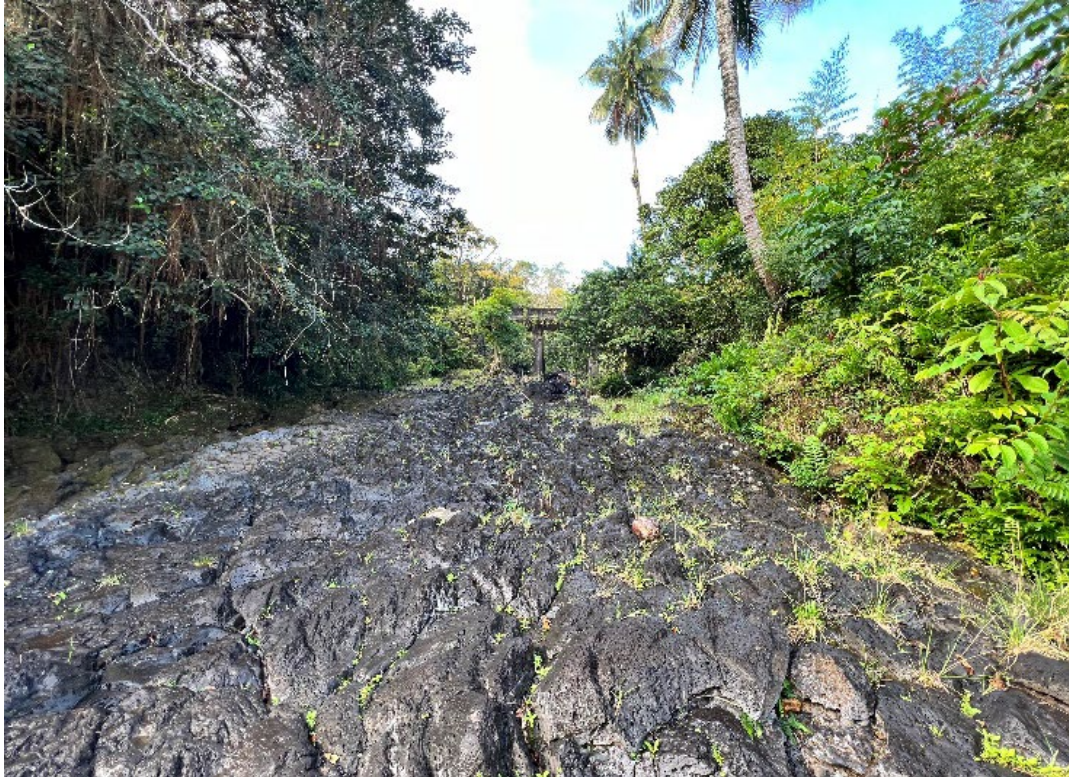
Photo 3-6. Bridge #40—Mokulehua Stream Bridge crossing the Kawakoe Stream (looking upstream from the makai side of the bridge)
