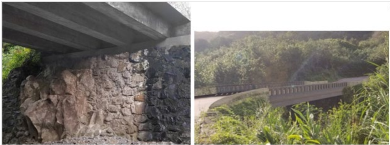
Rendering of Bridge #2—Kailua Stream Bridge on new foundation behind CRM Abutment to remain
