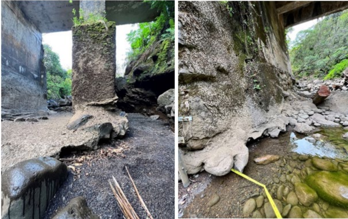
Figure 1-2. Undermining at Bridge #40—Mokulehua Stream Bridge and Bridge #8—Puohokamoa Stream Bridge
