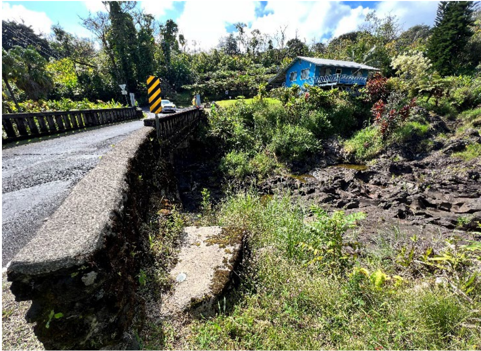
Photo 3-5. Bridge #39—Ulaino Stream Bridge crossing the Heleleikeoha Stream (looking along the mauka side of the bridge)
