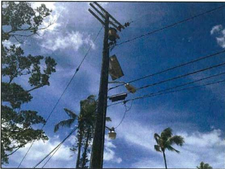
Photograph 18: View of pole-mounted transformer located east of Building No. 3 (residence).
