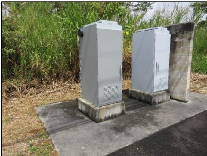
Photograph 12. A view of the Hawaii Electric Light Company (HELCO) street light and traffic signs closets east to parcel 007. The concrete pad is stained due to potential mildew (31 May 2023).
