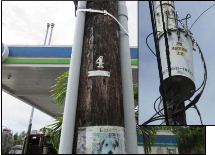
Photograph 7. A view of a pole-mounted transformer on an adjoining property (parcel 069) to the south of parcel 007 (31 May 2023).
