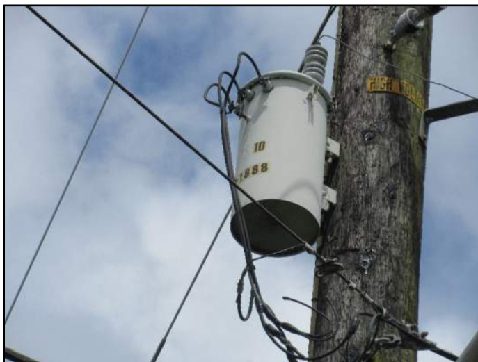
Photograph 18. A view of the pole-mounted transformer east of parcel 007 (31 May 2023).
