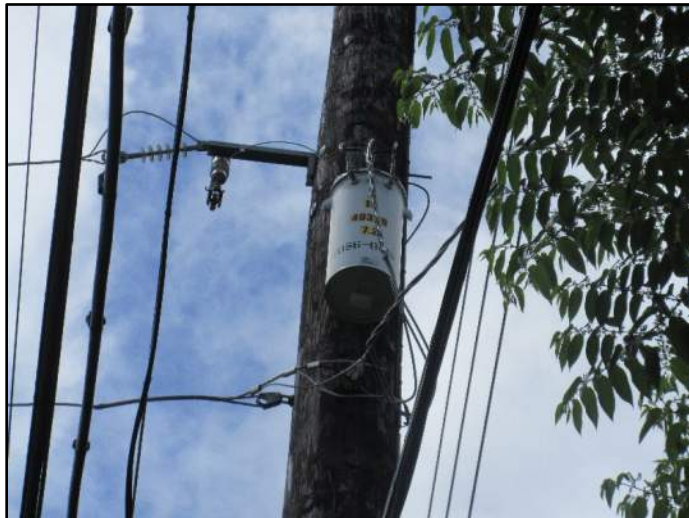
Photograph 14. A view of the pole-mounted transformer east of the subject property at parcel 007 (31 May 2023).
