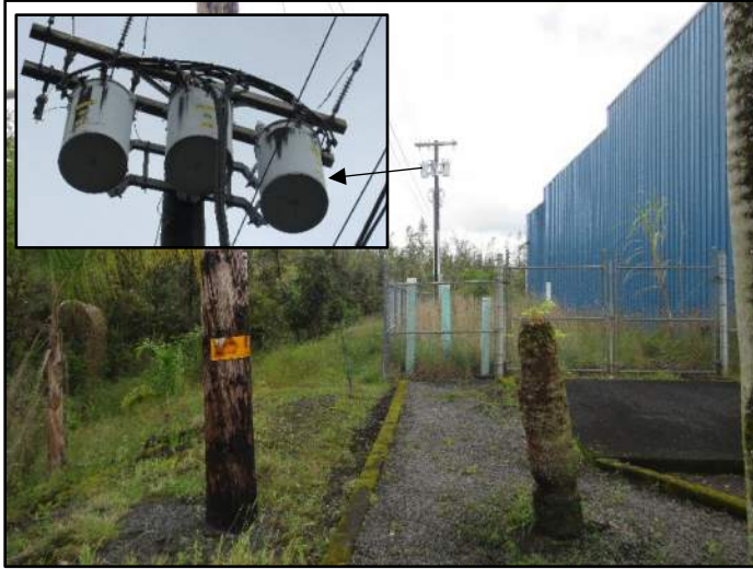
Photograph 22. A view of three pole-mounted transformers on the adjoining property to the north (parcel 080) (31 May 2023).
