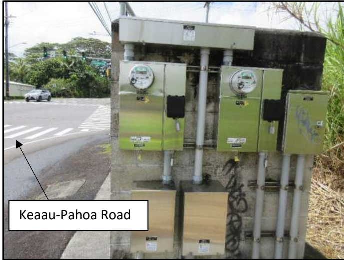
Photograph 13. A view of the back side of a concrete wall with street light and traffic sign meters as well as the HELCO gutter box and communication cabinet east of the subject property at parcel 007 (31 May 2023).
