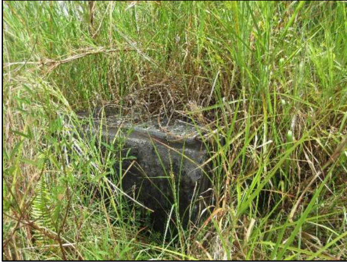
Photograph 10. A view of the concrete structure with drainage grate, located in the southern area of parcel 007 (31 May 2023).
