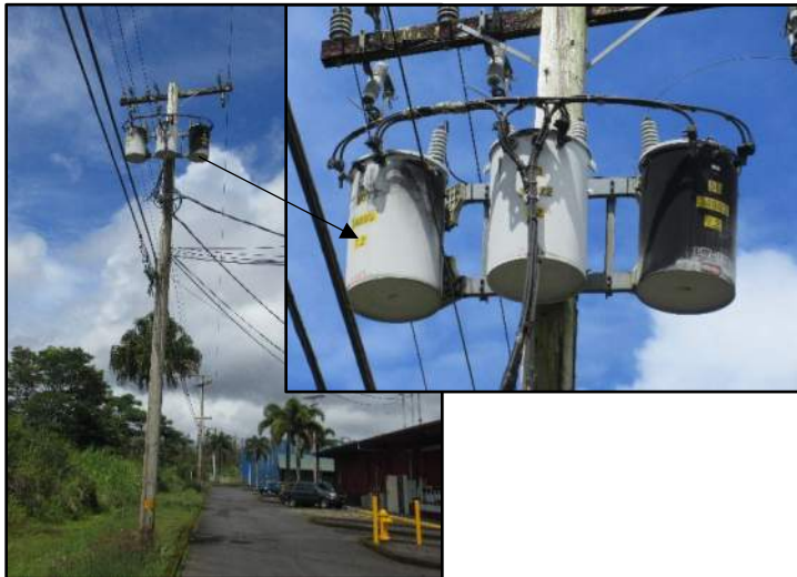
Photograph 20. A view of the three pole-mounted transformers on the adjoining property to the north (parcel 080) (31 May 2023).
