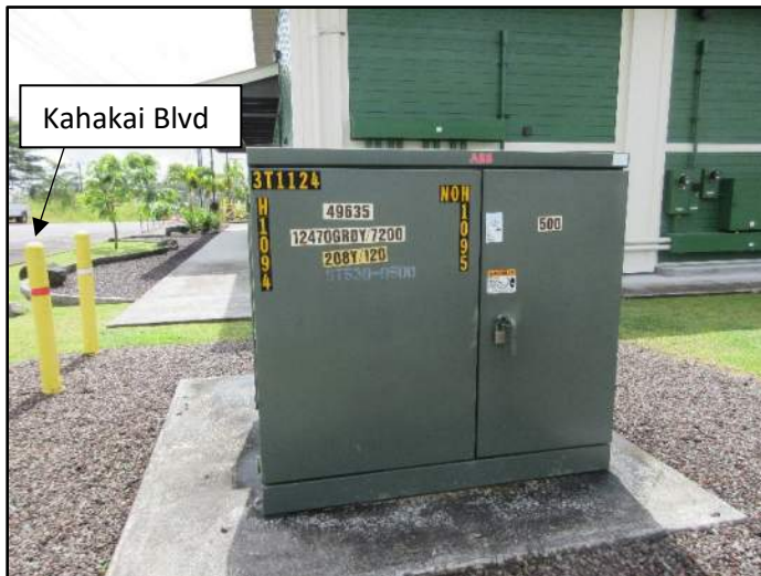
Photograph 8. A view of the pad-mounted transformer on the adjoining property (parcel 069) to the south of parcel 007. Stain on the concrete pad appears to be mildew (31 May 2023).
