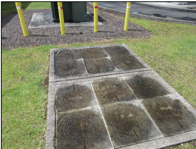
Photograph 9. A view of the cable manholes west of the pad-mounted transformer on the adjoining property, parcel 069. The concrete cap is stained due to rain/water and potential mildew (31 May 2023).
