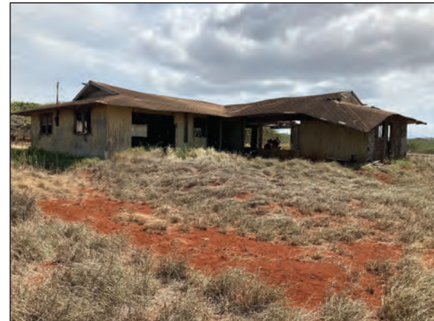
Figure 39. Photo L: View of the abandoned house in the 4.7-acre TMK: [2] 5-2-026:014 parcel
