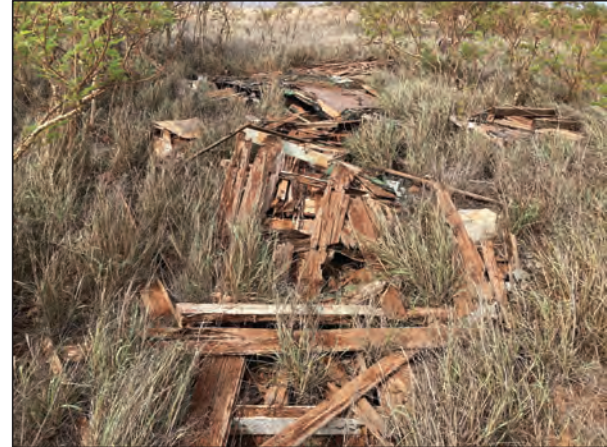
Figure 31. Photo E: View of collapsed structure in the 31.7-acre TMK: [2] 5-2-005:031 parcel, view to southwest
