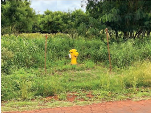
Picture 8. Site #7 includes new hydrant and valve locations.
