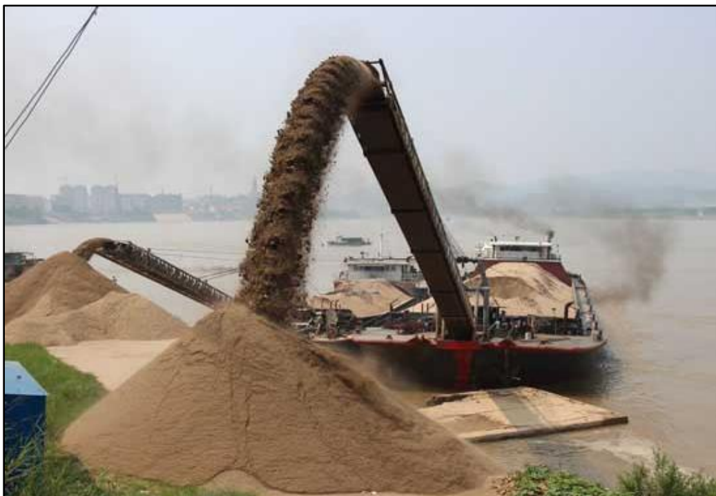
Figure 5-15 Barge-mounted conveyor system
