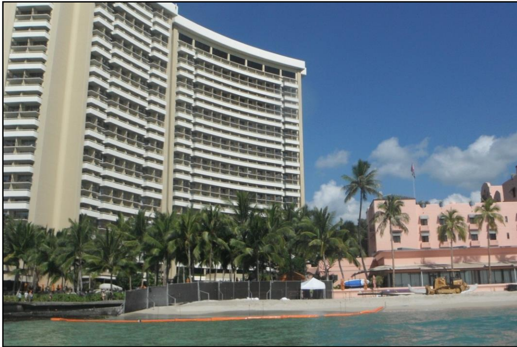
Figure 5-17 Example: floating silt curtain and small bulldozer used for sand placement in the 2012 Waikiki Beach Maintenance project.
