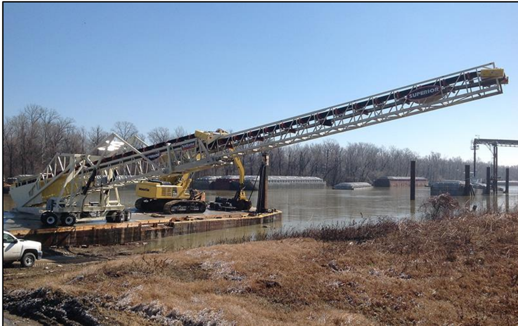
Figure 5-14 Barge-mounted conveyor system
