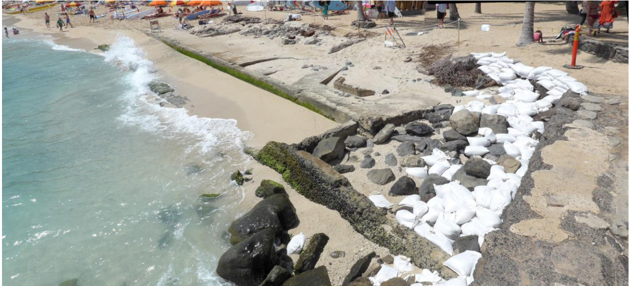
Photo 4. Concrete foundation exposed by erosion at the Diamond Head end of the Royal Hawaiian sector, May 17, 2017. Photo courtesy of Matt Bell.
