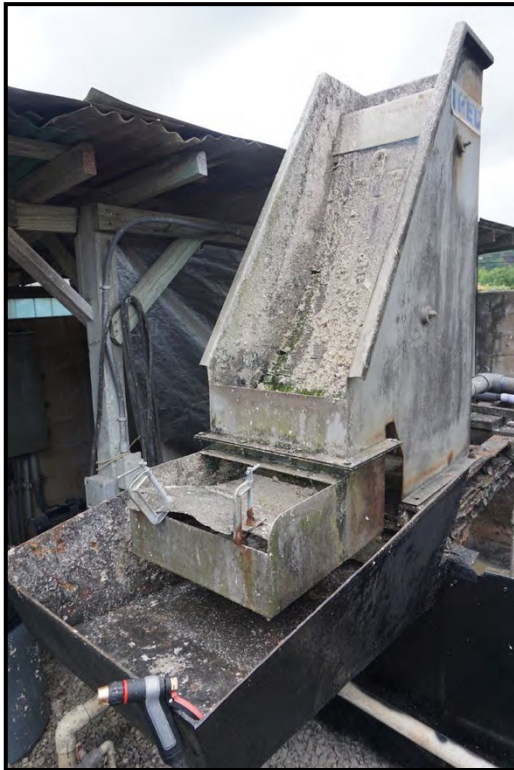
Photo9: Existing WWTP Communitor within WWTP enclosure. Facing southwest.
