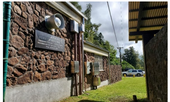
View of existing Round Top Radio facility and overhead power lines facing mauka
