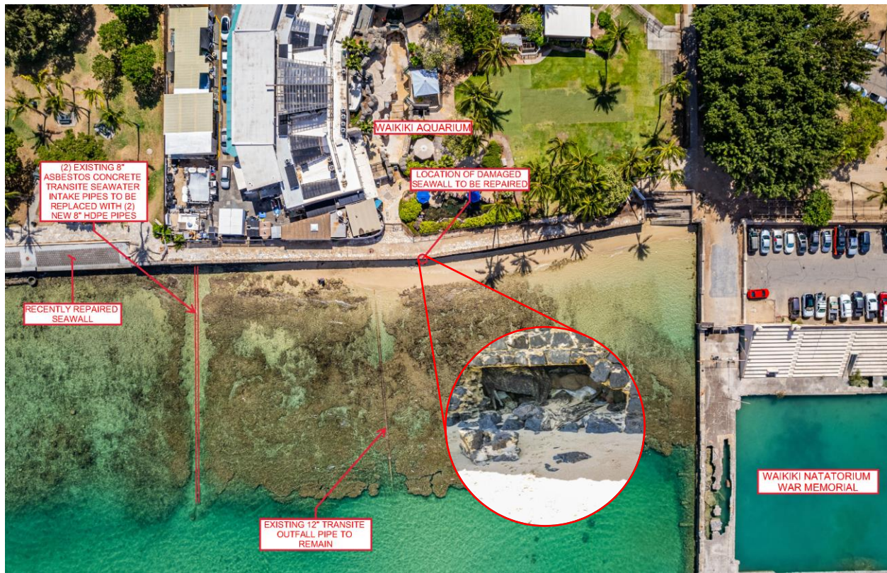
Figure 3-6: Location of Damaged Seawall to be Repaired
