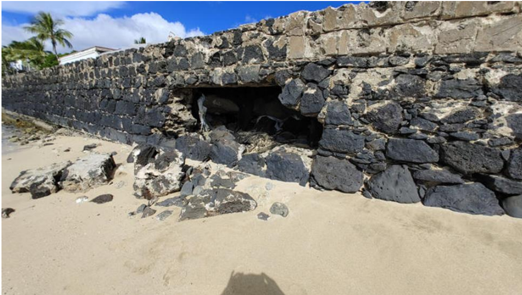
Figure 2-11a: Seawall In Need of Repair
