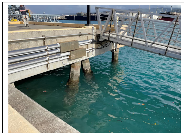
Sideview of existing Berth G with concrete decking supported by vertical and batter piles. The proposed pile-supported pier is likely to be similar in construction.
