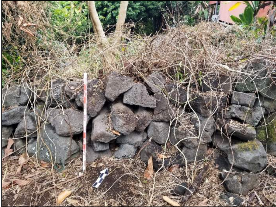
Figure 100. Photo showing construction of SIHP # -31124 Feature A mauka-makai wall; view to northwest
