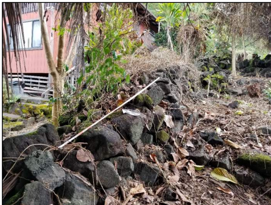
Figure 99. Photo showing a portion of SIHP # -31124 Feature A mauka-makai wall; view to northeast
