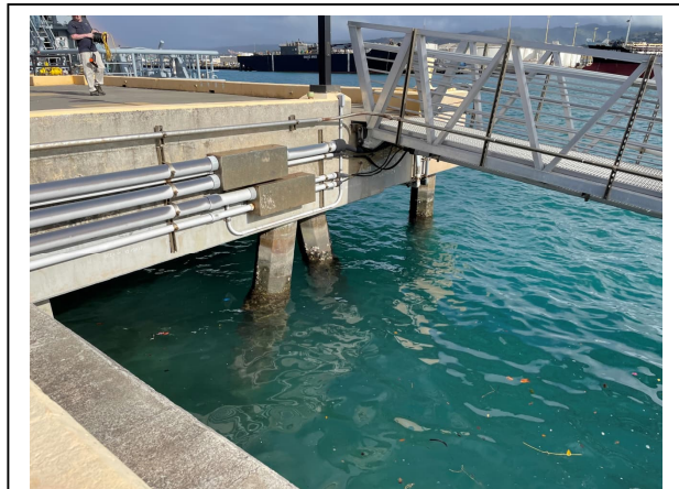
Sideview of existing Berth G with concrete decking supported by vertical and batter piles. The proposed pile-supported pier is likely to be similar in construction.
