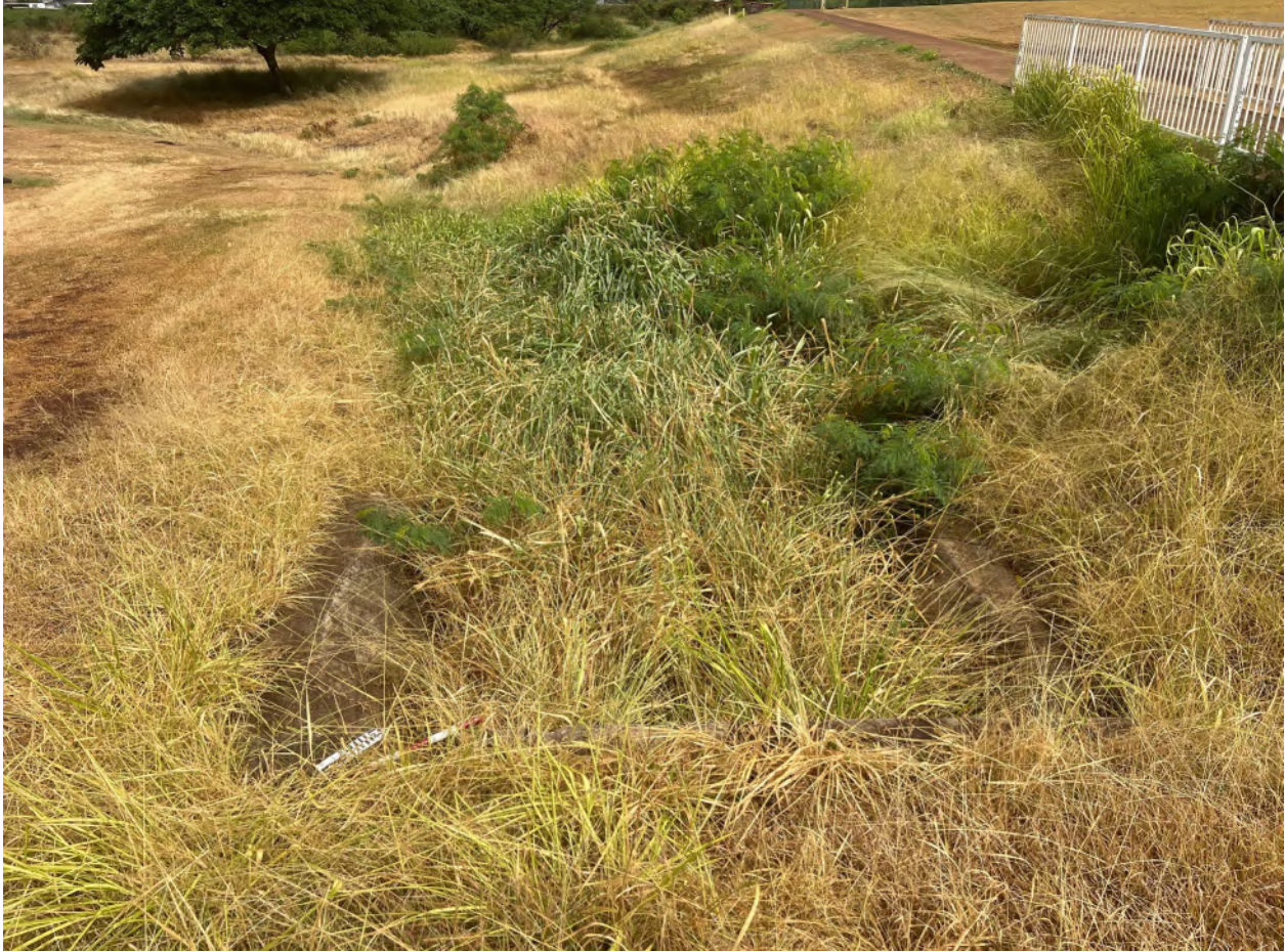
Photo 6 – Another view of concrete culvert head wall (see previous two photographs) facing northwest
