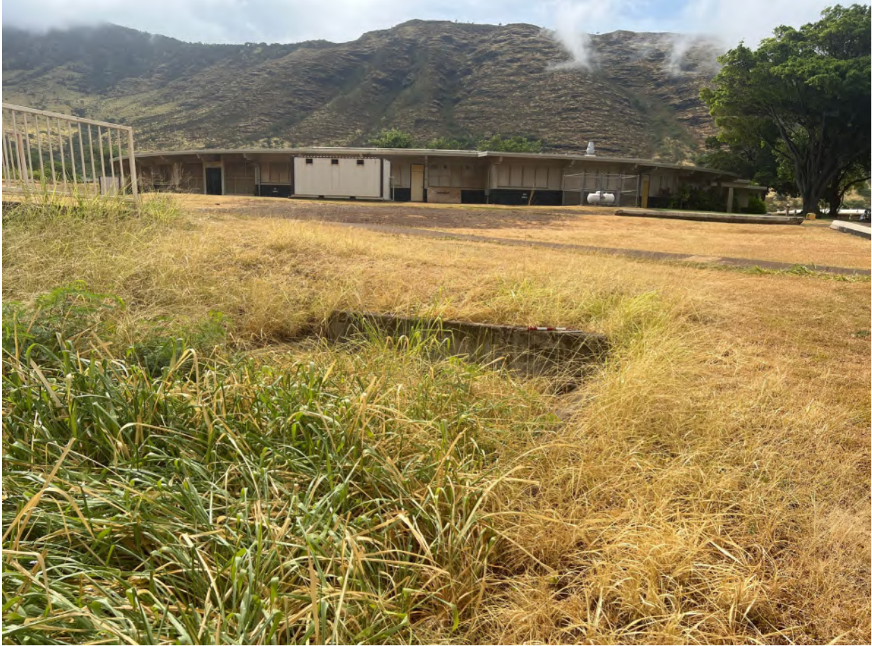
Photo 5 – Overview of concrete culvert head wall (see previous photograph) facing east
