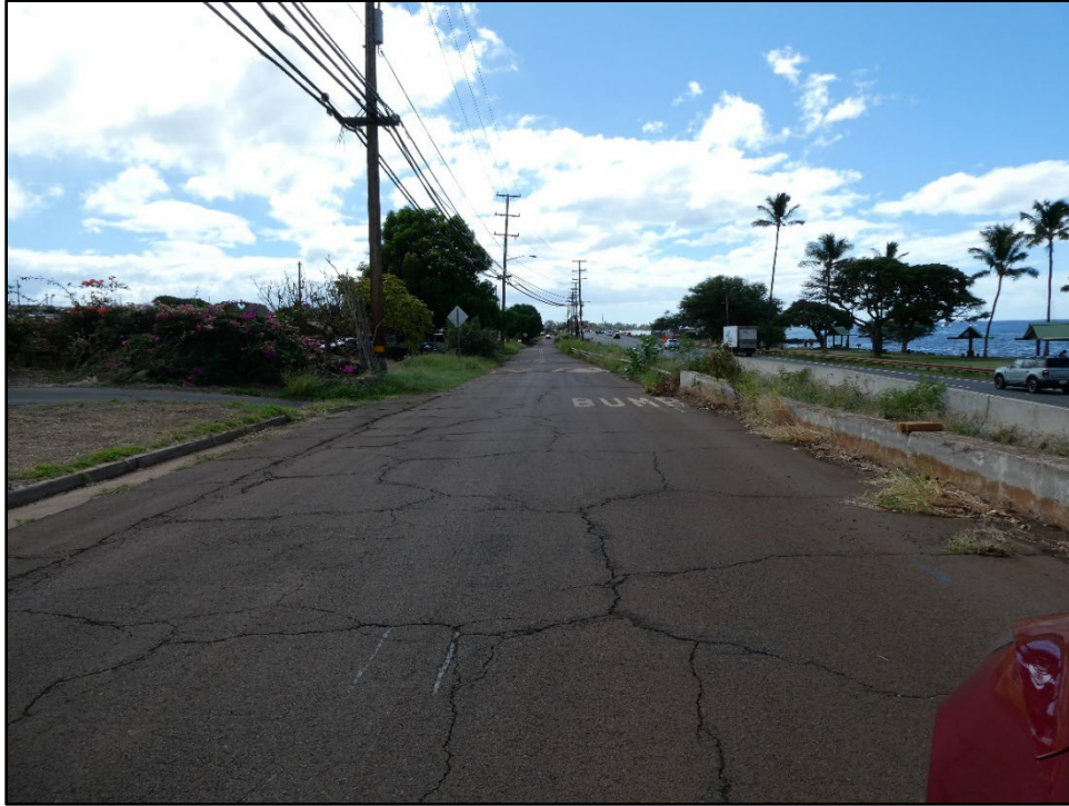
Figure B-11. View south along Malo Street and western APE boundary between Kekai and Kalani Roads.
