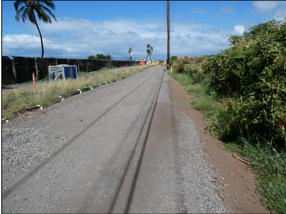
Figure B-21. View north along Malo Street and western APE boundary near the Lahaina 3 Pump Station.
