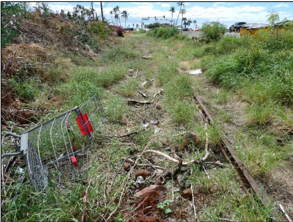
Figure 21. Newly identified segment of SIHP Site 50-50-03-08887 (railroad) trending along Malo Street north of the Fleming Road-Honoapi'ilani Highway junction outside the western boundary of the APE, view to the north.
