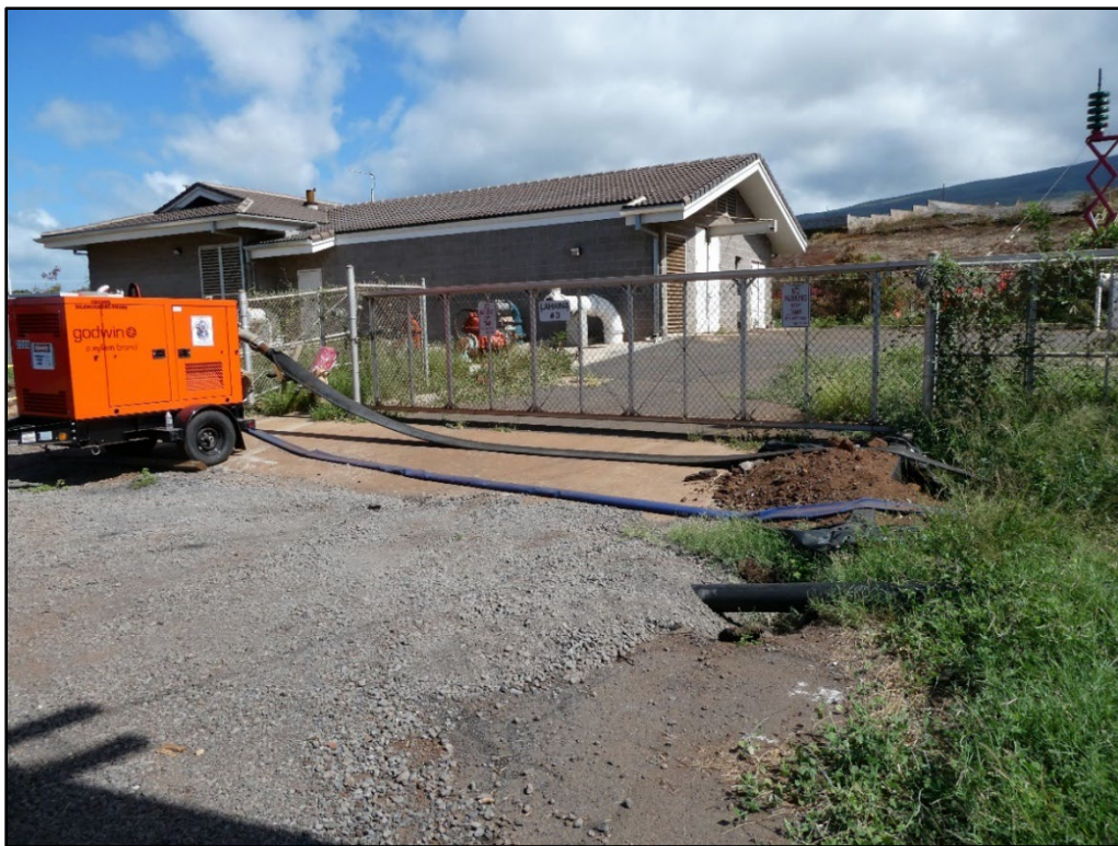
Figure 23. Lahaina 3 Pump Station near the southernmost portion of the APE, view to the northeast.
