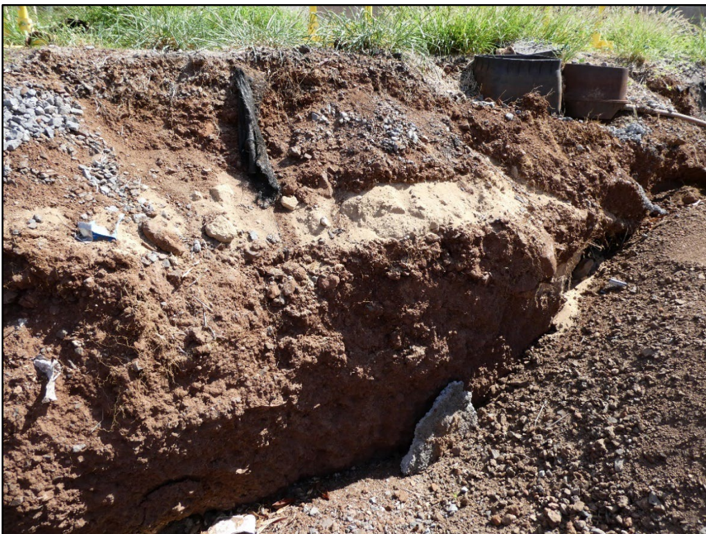
Figure 27. Sand fill sediments observed in an open exposure near the Lahaina 3 Pump Station, view to the southeast.
