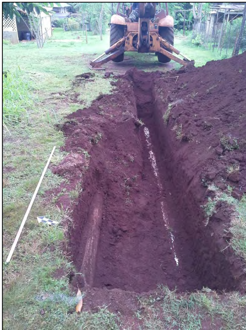
Figure 31. T-5, overview of utilities; view to east
