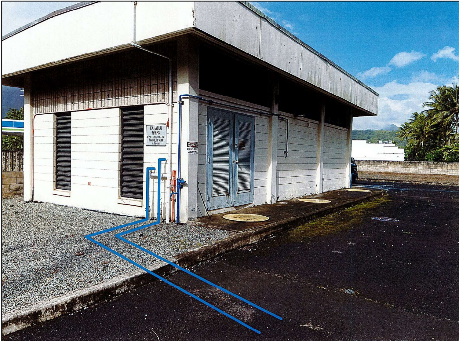
Figure 6. Indicated route of underground fuel piping approaching the Kahaluu WWPS building (Okahara and Associates, Inc.; courtesy of client)
