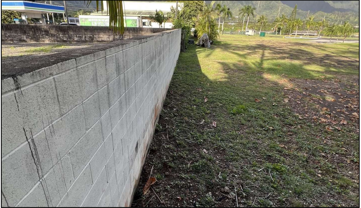
Figure 34. Photo E: View of north wall of the WWPS property showing raised ground surface, view to west
