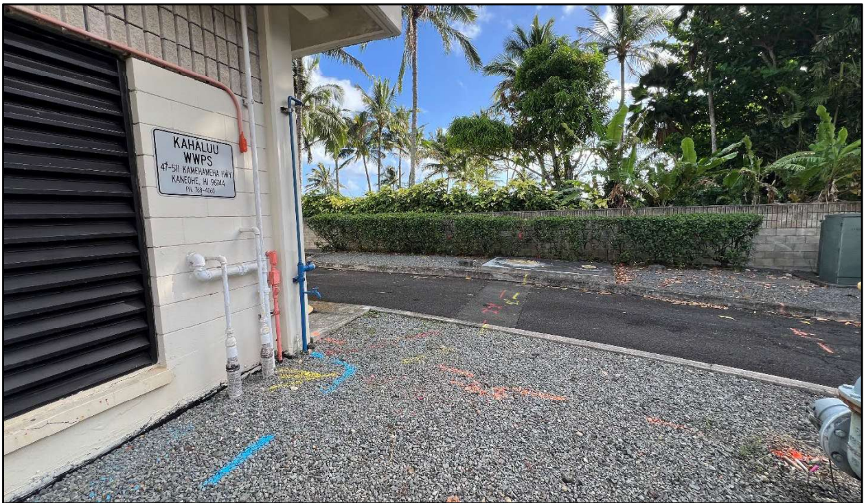
Figure 35. Photo F: View of south end of the WWPS property showing numerous utility lines, note the existing underground storage tank in center of photograph, view to east
