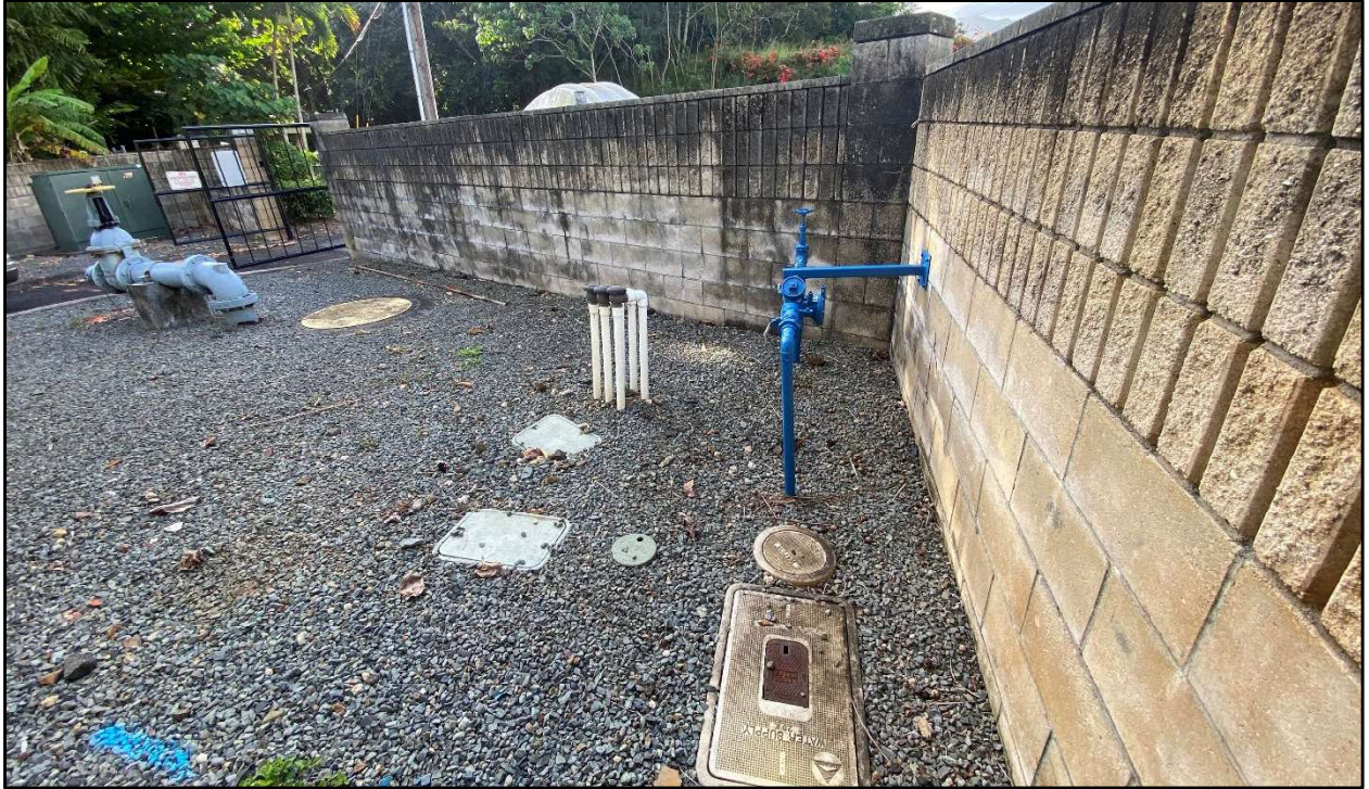
Figure 36. Photo G: View of south end of the WWPS property showing numerous utility lines, view to south
