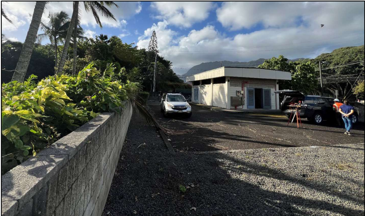
Figure 33. Photo D: View east side of the WWPS property where new underground line will extend from the existing underground storage tank in background to the new aboveground storage tank location in foreground, view to south
