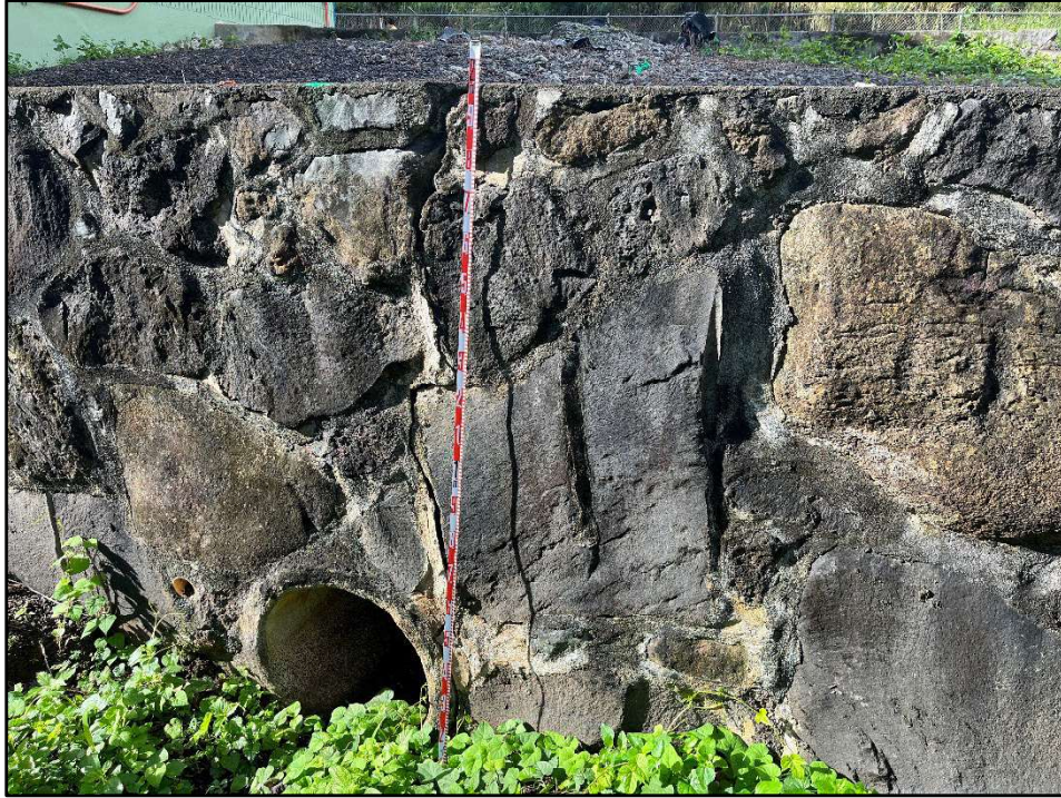
Figure 50. Photo S: Close-up of northeast retaining wall at the Kukanono WWPS facility under evaluation for repair/replacement showing cracking (to left of tape measure), view to southwest
