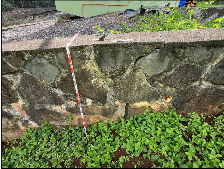
Figure 48. Photo Q: Close-up of northwest retaining wall at the Kukanono WWPS facility under evaluation for repair/replacement showing cracking (to right of tape measure), view to southeast
