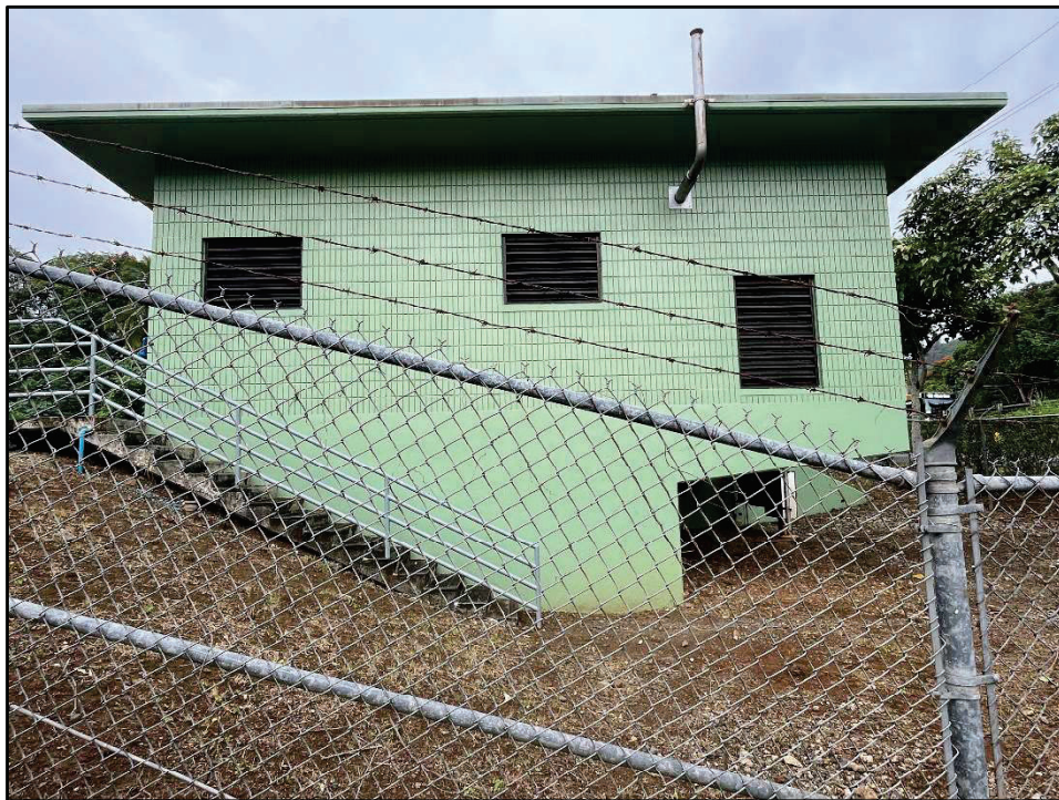
Figure 39. Photo H: View of the east side of the existing Pump Station building (from outside the enclosure), view to west
