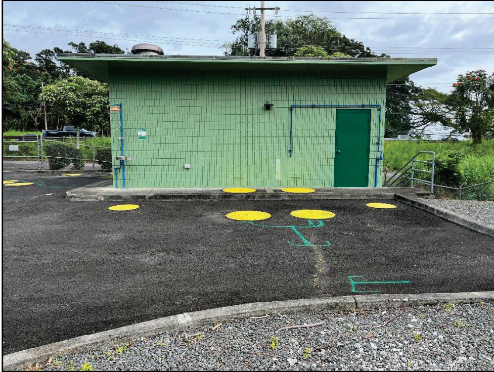
Figure 40. Photo I: View of the south side of the existing Pump Station building, view to north
