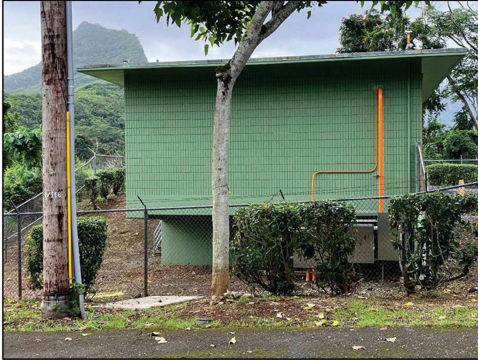
Figure 38. Photo G: View of the north side of the existing Pump Station building (from Auloa Road), view to south
