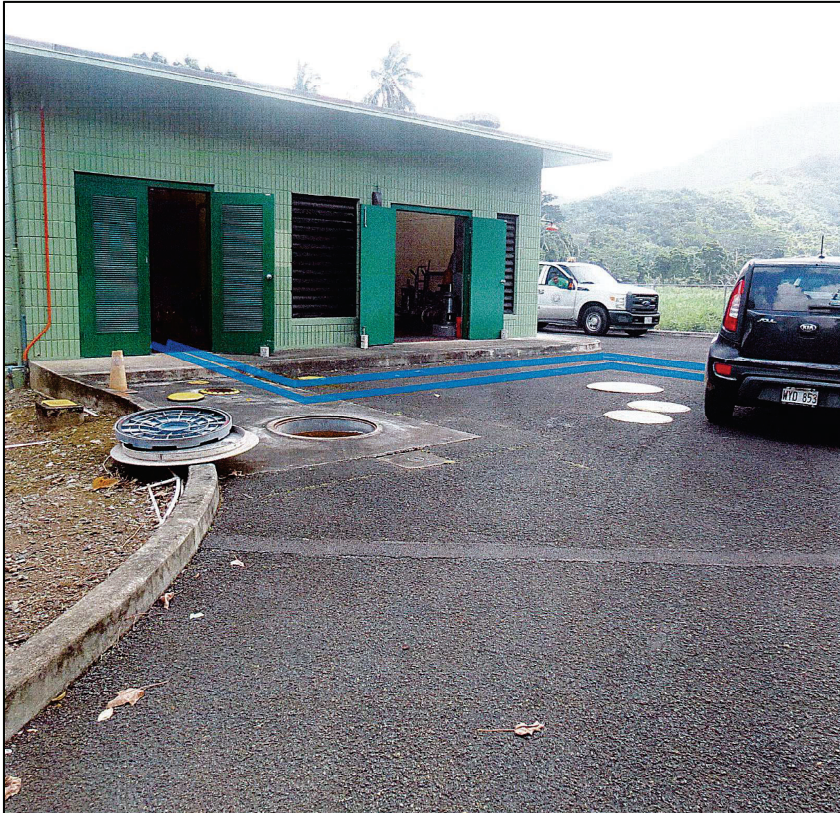
Figure 6. Photograph showing the location of new underground fuel piping as it enters existing pump station building, view to south (Okahara and Associates, Inc.; courtesy of client)
