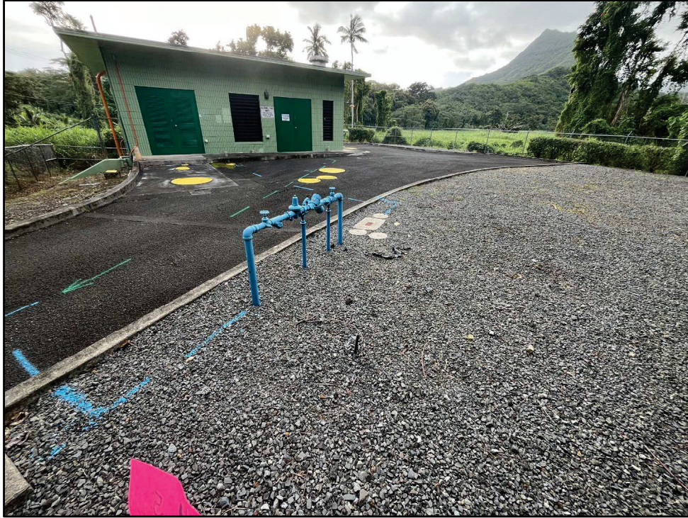
Figure 36. Photo E: View of the Maunawili Park WWPS from the northwest corner of the enclosure, the proposed AST would be at the right, view to southeast
