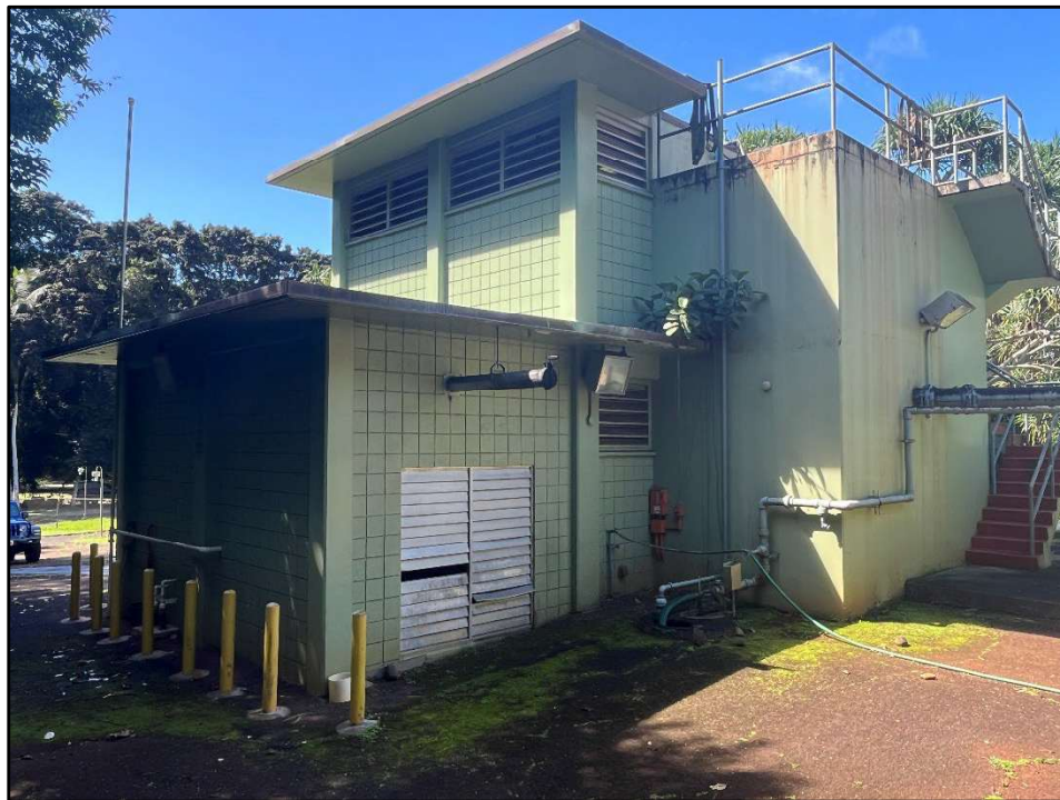
Figure 33. Photo H: View of the northeast side of the Pacific Palisades WWPS Pump Station building, view to southwest
