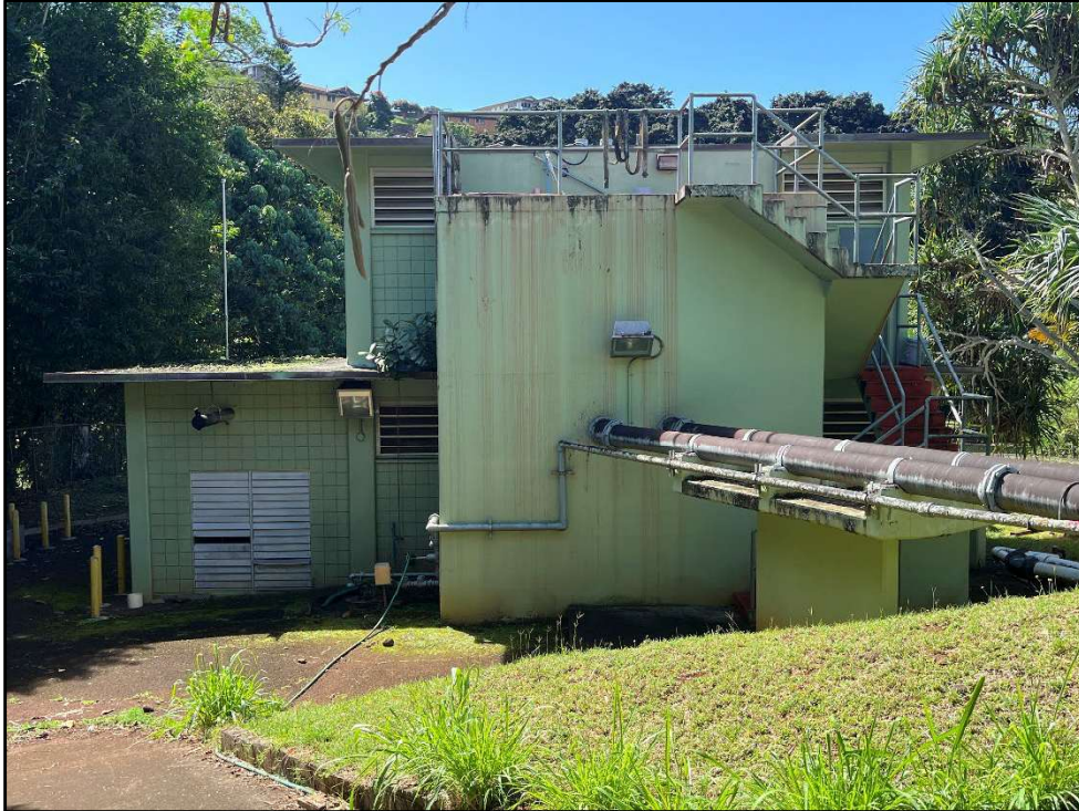
Figure 32. Photo G: View of the back (northwest side) of the Pacific Palisades WWPS Pump Station building, view to northwest
