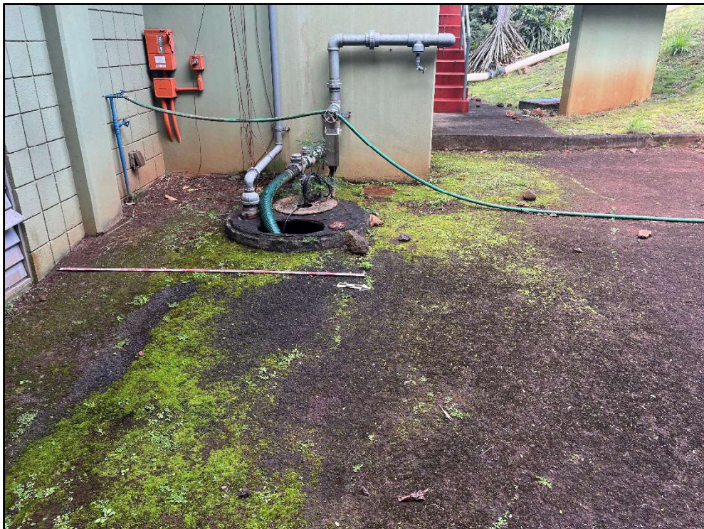
Figure 39. Photo N: View of area for proposed fuel supply/return piping, view to west
