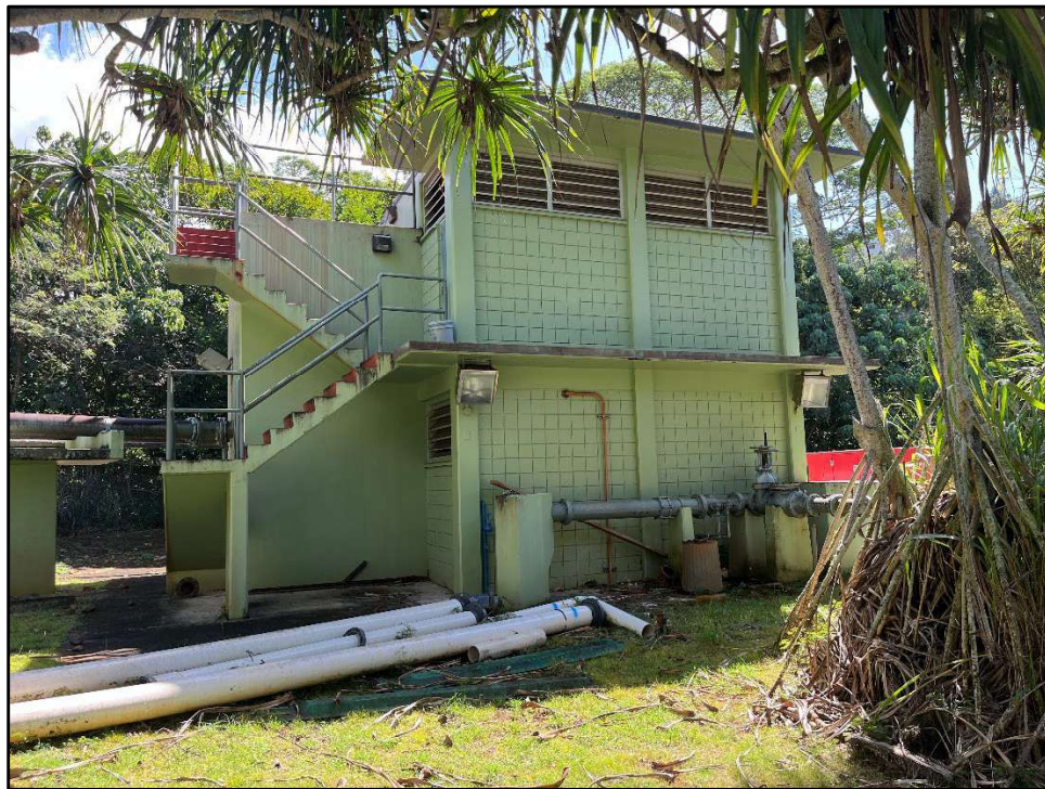
Figure 31. Photo F: View of the southwest side of the Pacific Palisades WWPS Pump Station building, view to southeast
