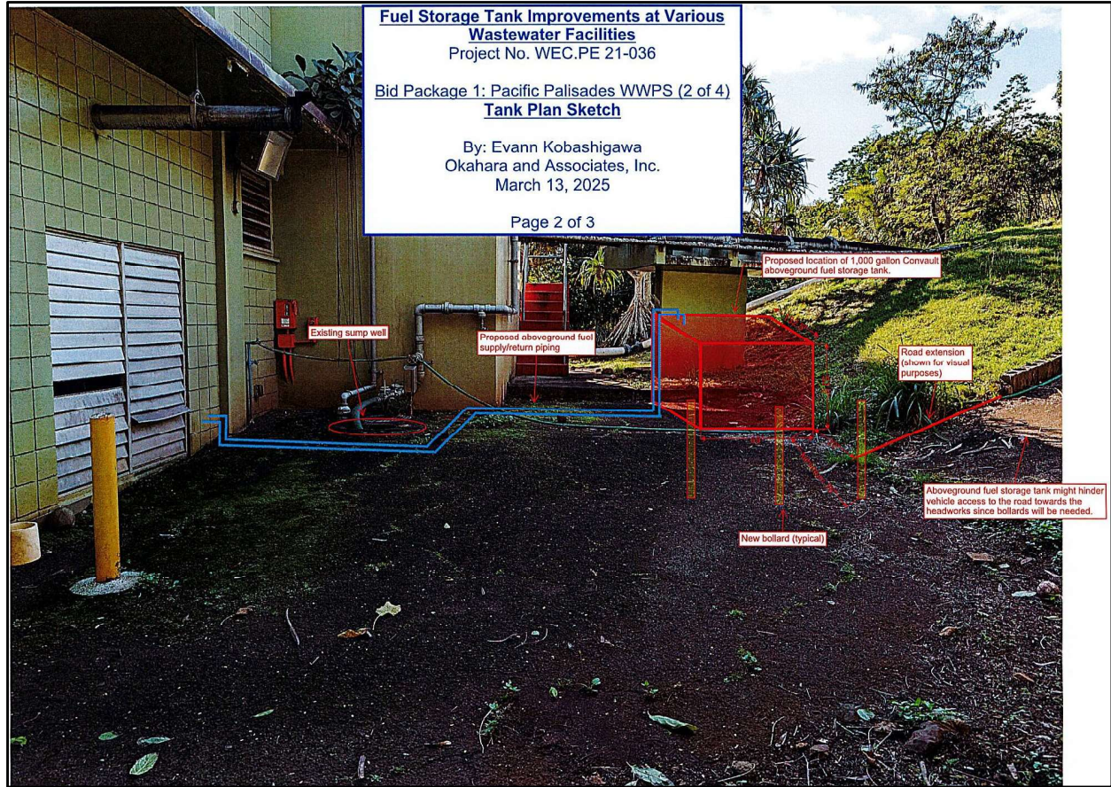
Figure 5. Photograph showing the proposed location of the new 1,000-gallon Convault above ground fuel storage tank and proposed fuel supply/return piping north of the Pacific Palisades WWPS pump station building (Okahara and Associates, Inc.; courtesy of client)
