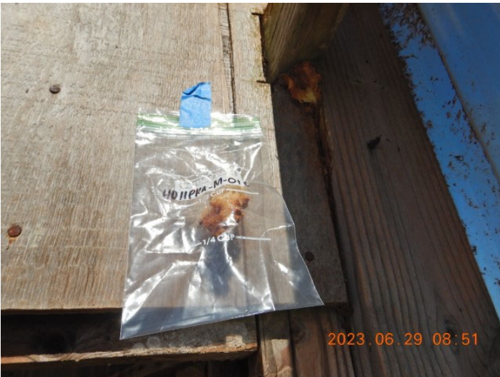
Photo 27 - 4011PKA-M-01C (Close-up) [BB\DSCN9812.JPG]
