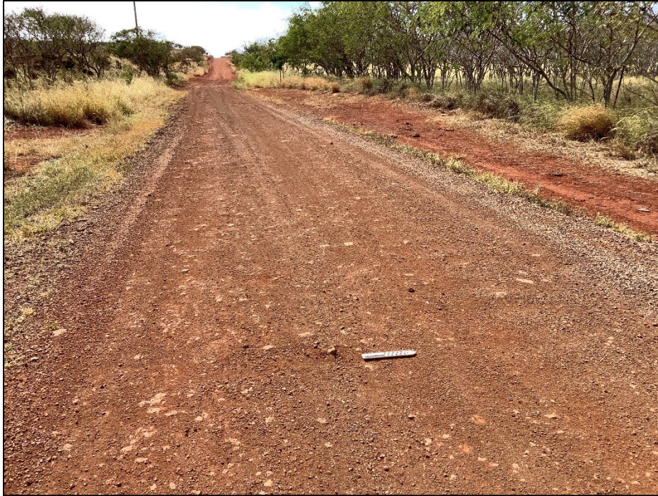
Figure 38. General view of a portion of Mo'omomi Avenue within the roadway and drainage improvements portion of the project area, view to west
