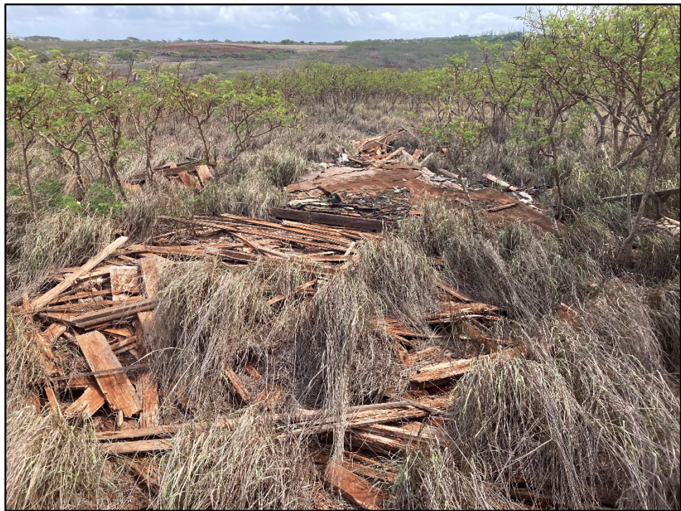
Figure 32. Photo F: View of collapsed structure in the 31.7-acre TMK: [2] 5-2-005:031 parcel, view to northeast
