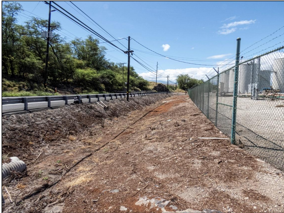
Figure 3. Drainage feature on the makai side of Kawaihae Road adjacent to harbor security fence.
