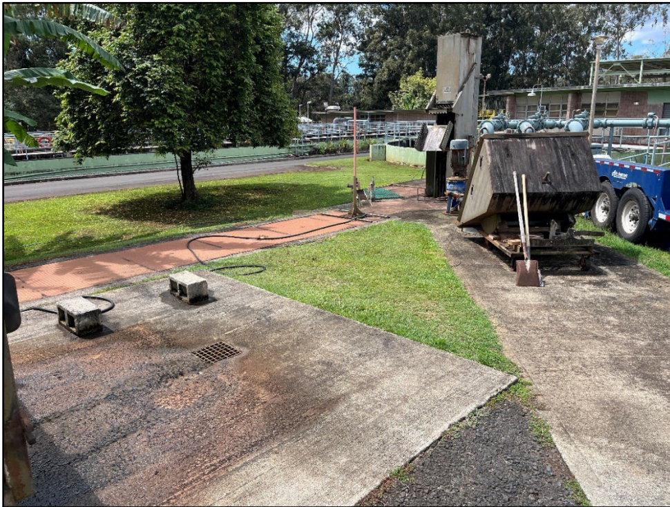
Figure 39. Photo N: General view from the central portion of the Wahiawa WWTP, view to southwest
