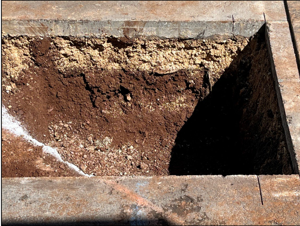
Figure 32. Photo G: Open in-progress excavation within 20 m of project area, view to northwest
