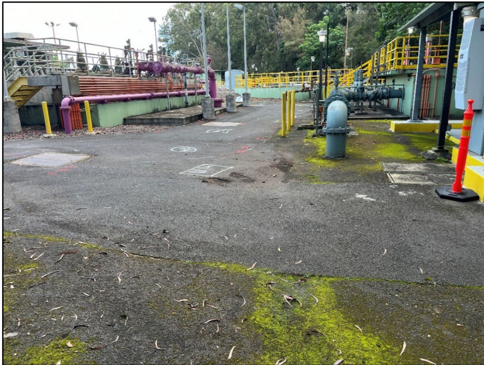
Figure 35. Photo J: General view of the Wahiawa WWTP from the south corner, view to northeast
