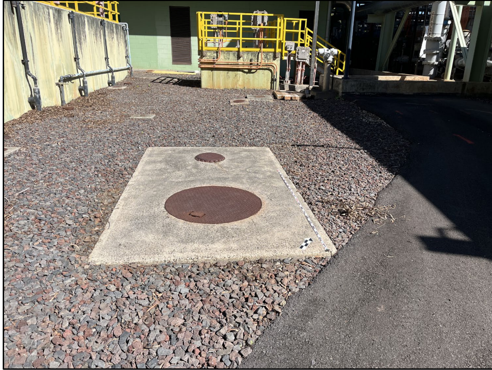
Figure 26. Photo A: View of the immediate area of the 6,000-gallon diesel UST (at cement slab) to be removed (proposed AST area in background), view to northwest
