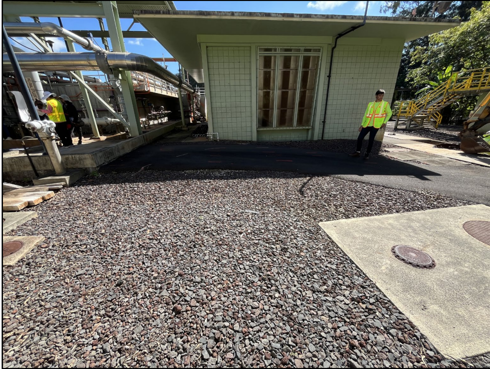
Figure 30. Photo E: Indicated route for fuel piping to generator building (in background), view to east
