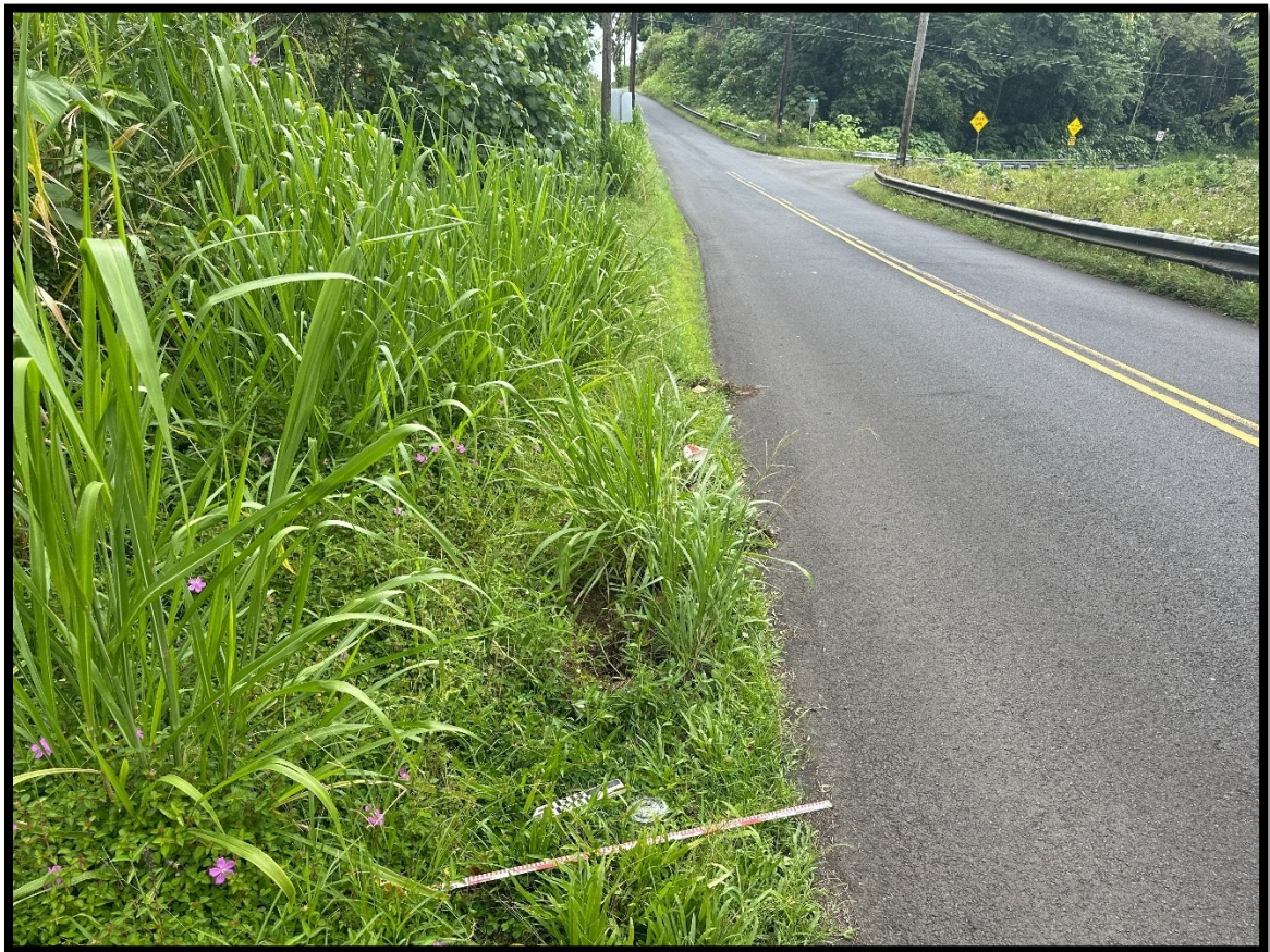
Figure 20. Overview photo of Kilauea Avenue south of the 4 Mile Bridge looking toward Hale Manu Drive
