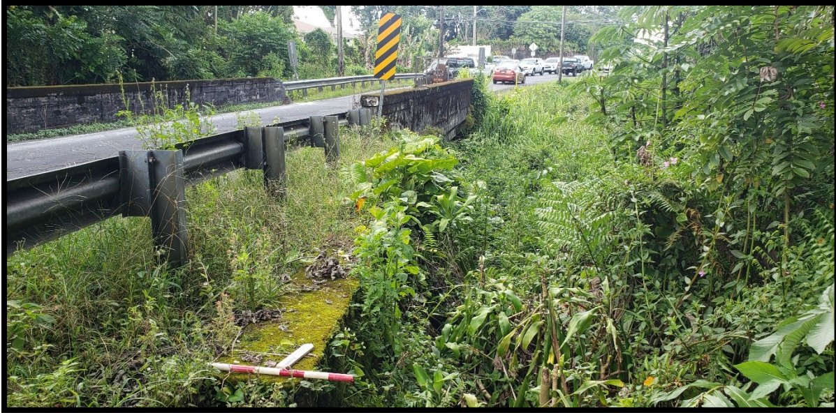
Figure 17. Overview photo of the western side of the 4 Mile Creek Bridge, looking south
