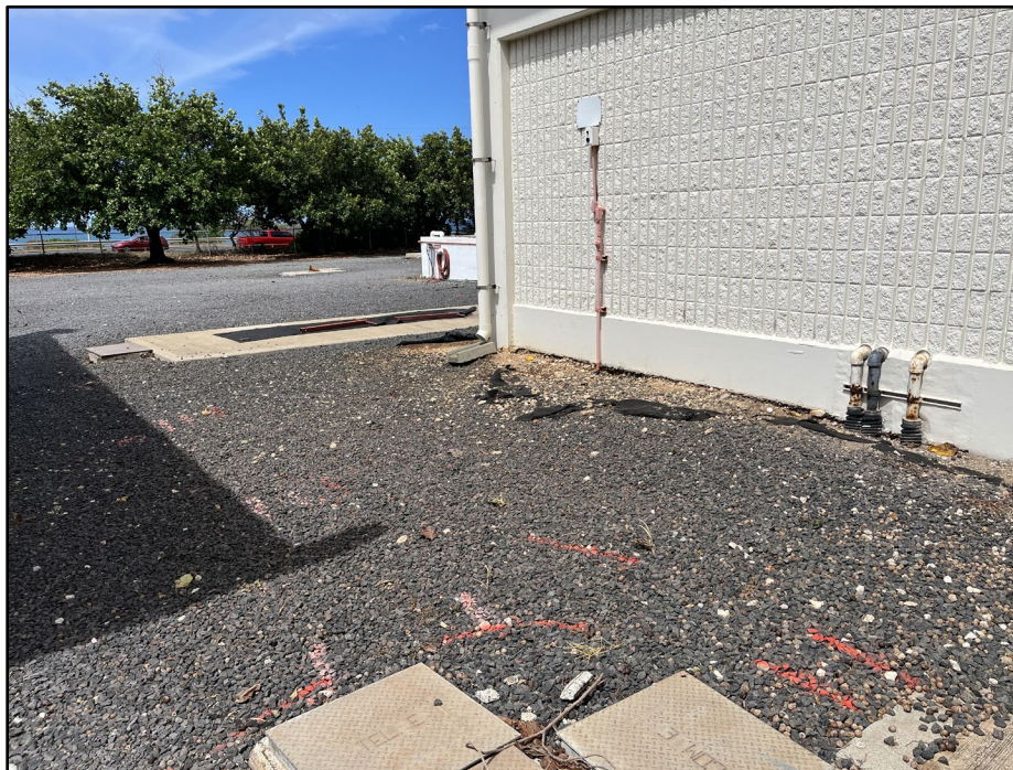
Figure 35. Photo D: View of the location of the south end of a new 6,000-gallon diesel AST at the location of a to-be-removed UST (under concrete slab) and new above ground fuel piping route connection to the southwest corner of the Generator Building (at center of photo) , view to northwest
