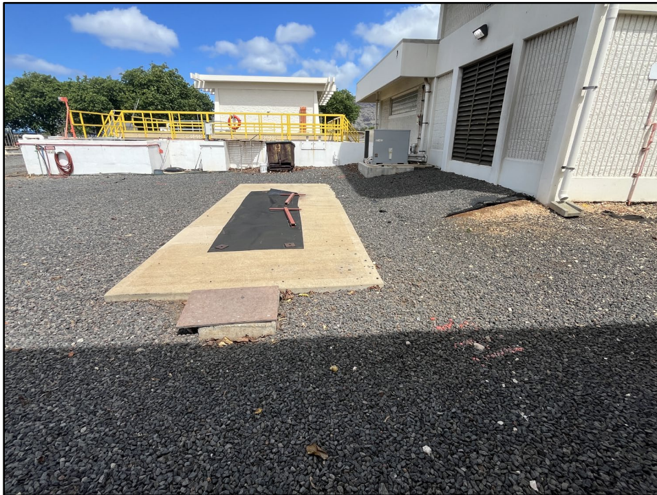
Figure 33. Photo B: View of the location of a new 6,000-gallon diesel AST at the location of a to-be-removed UST (under concrete slab), view to northwest
