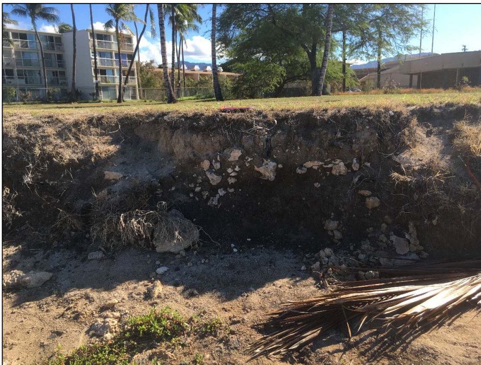
Figure 35. Exposed eroded coastal bank, showing coral/soil fill layers, view northeast
