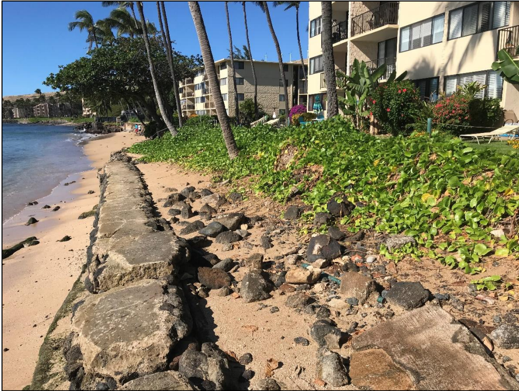
Figure 4-19 Cracking along concrete cap
