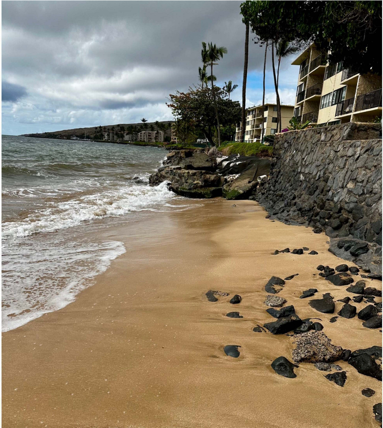
Figure 1 - Photo dated January 6, 2025 looking east to west with Hono Kai Seawall on the right of picture and Kanai A Nalu seawall (Zone 3) at the distant end of sandy beach. Note the natural sand along the shoreline at mid-tide extending approximately 10 feet from Hono Kai seawall. High risk of complete and permanent erosion of the beach with a setback at Kanai A Nalu.
