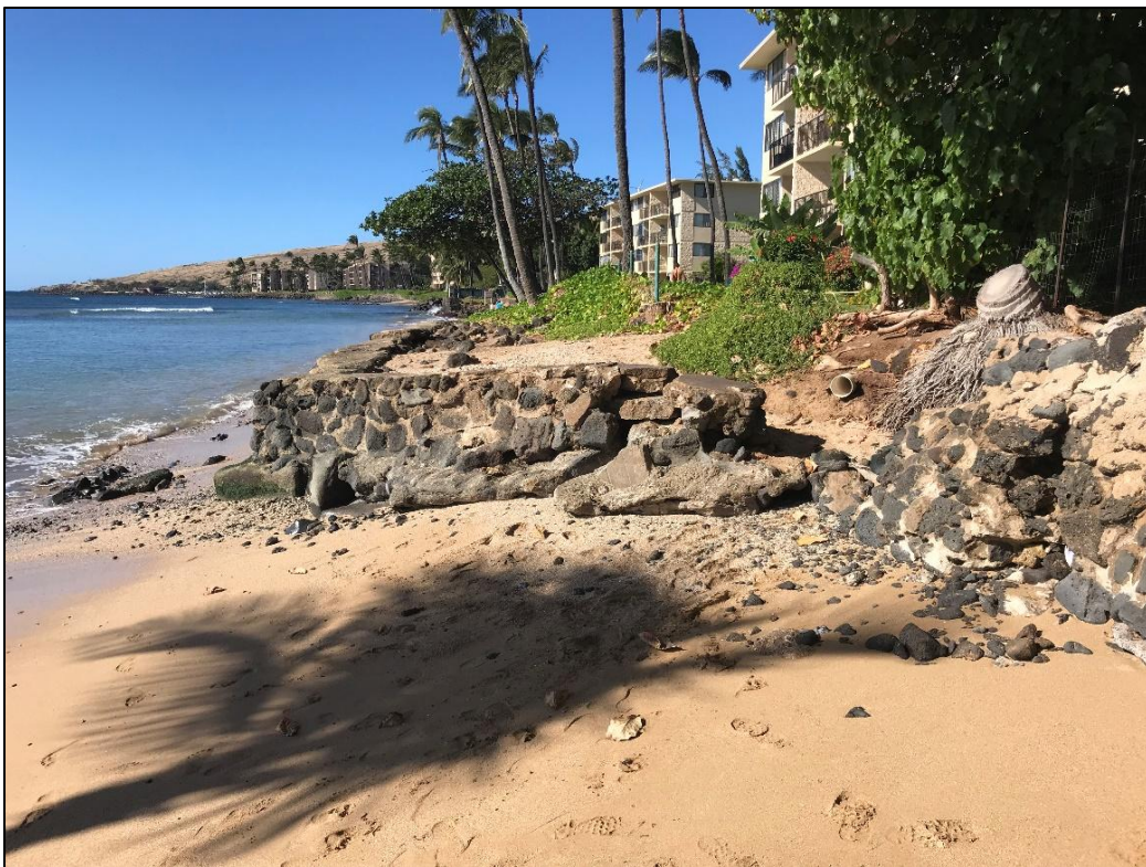
Figure 4-22 Damaged wall section at east end (adjacent seawall is also damaged)
