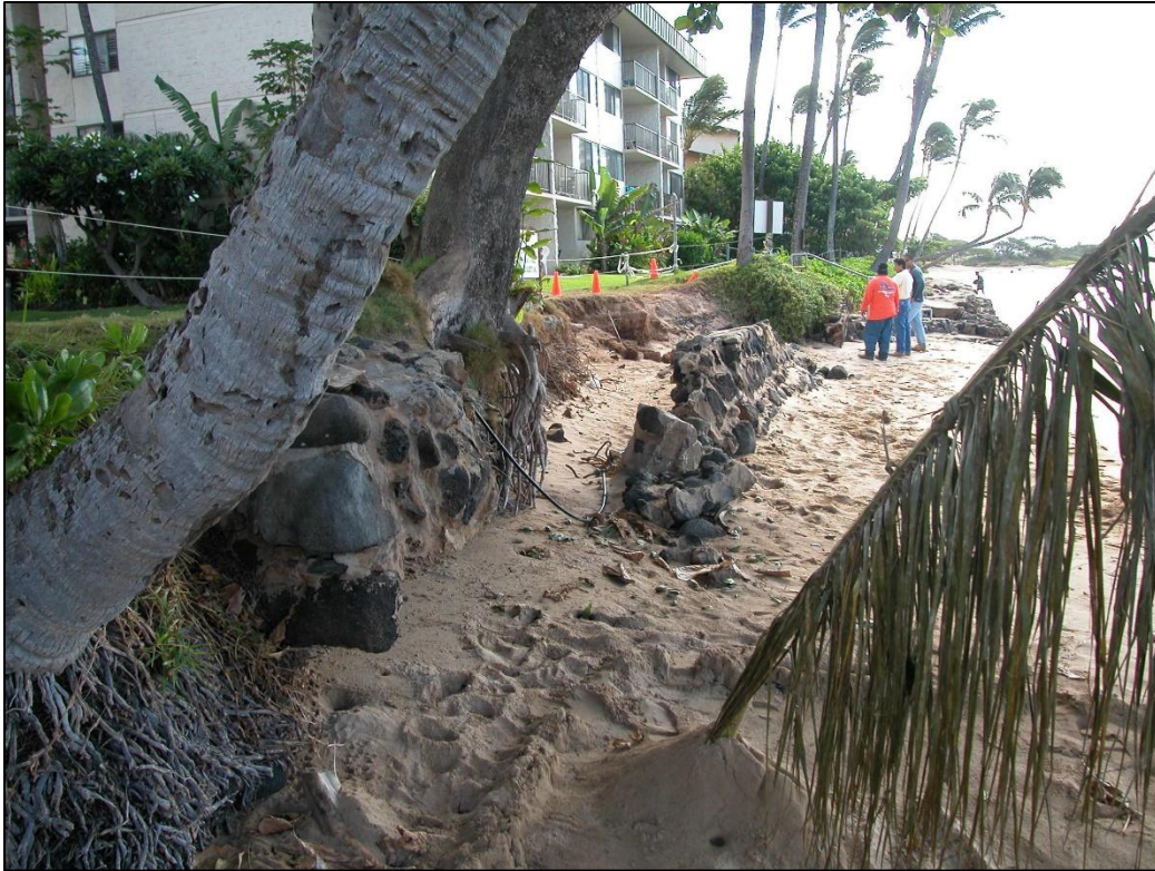
Figure 4-14 Failed seawall section (2009)
