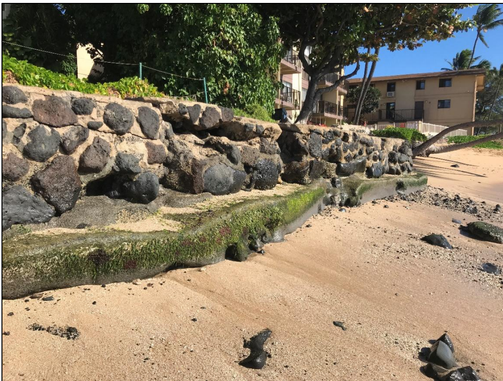
Figure 4-20 Cracking and dislodged stones on seawall face
