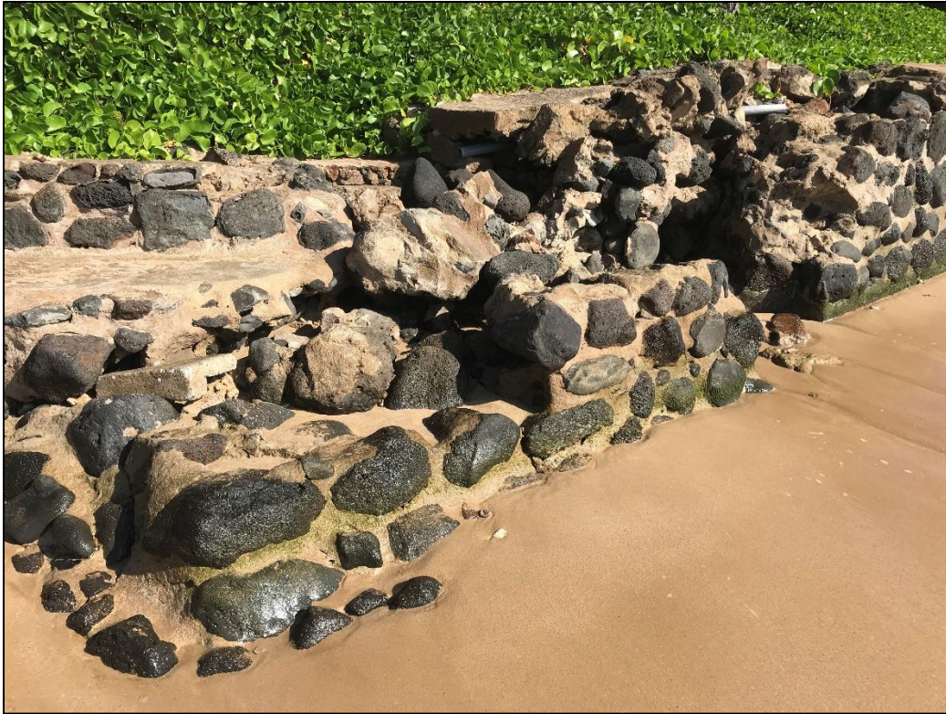
Figure 4-21 Damaged wall section east of CRM stair
