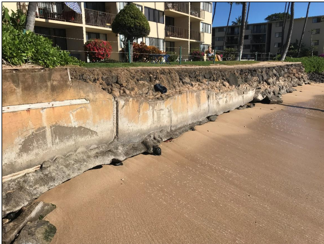
Figure 4-7 Undermining along toe of seawall
