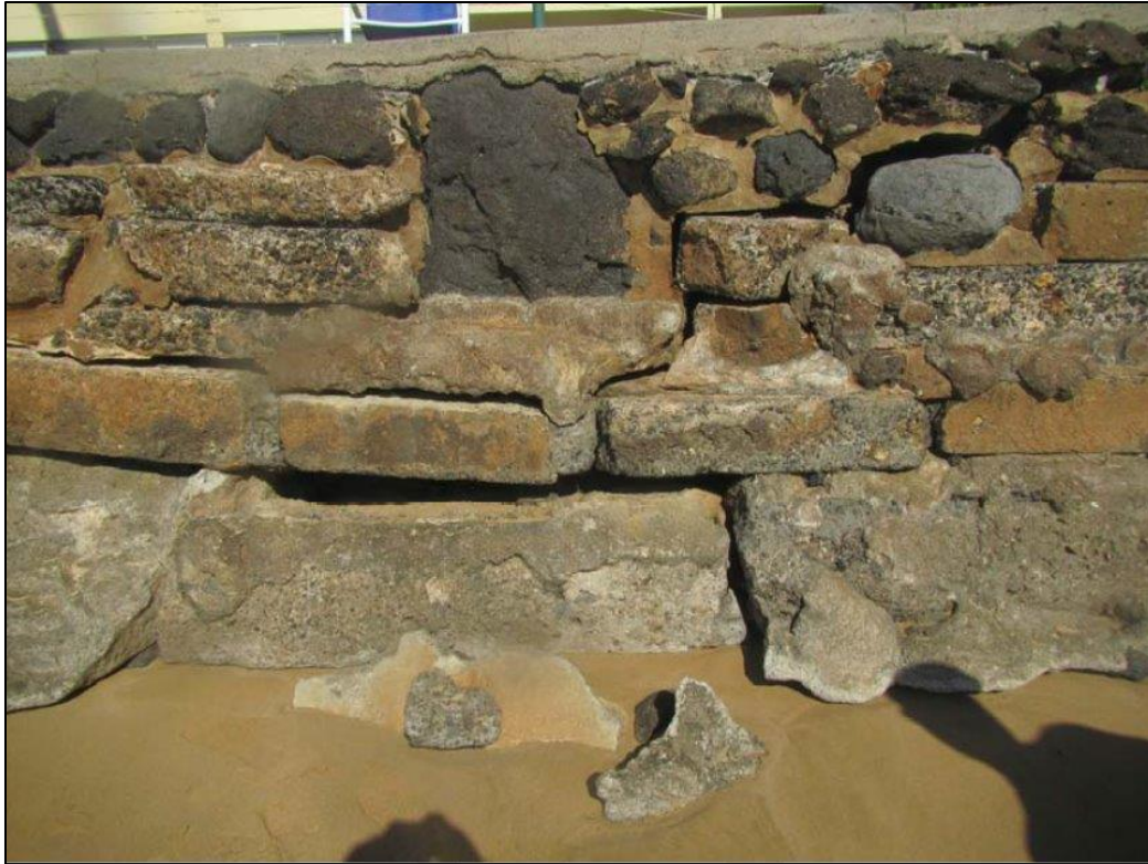
Figure 4-6 Cracks, mortar separation, and voids
