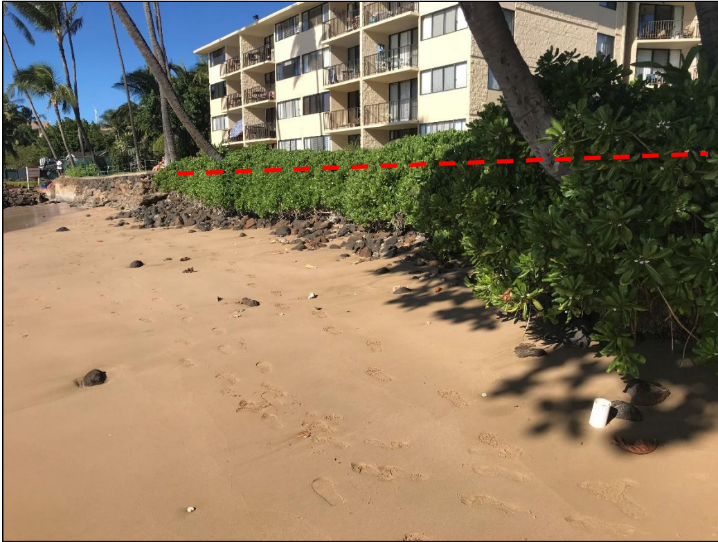
Figure 4-10 Approximate location of erosion scarp (dashed line)
