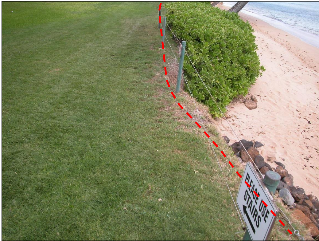
Figure 4-12 Erosion scarp along edge of lawn
