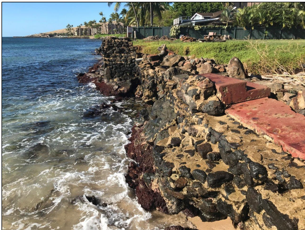
Figure 4-9 Damaged seawall on west adjacent property
