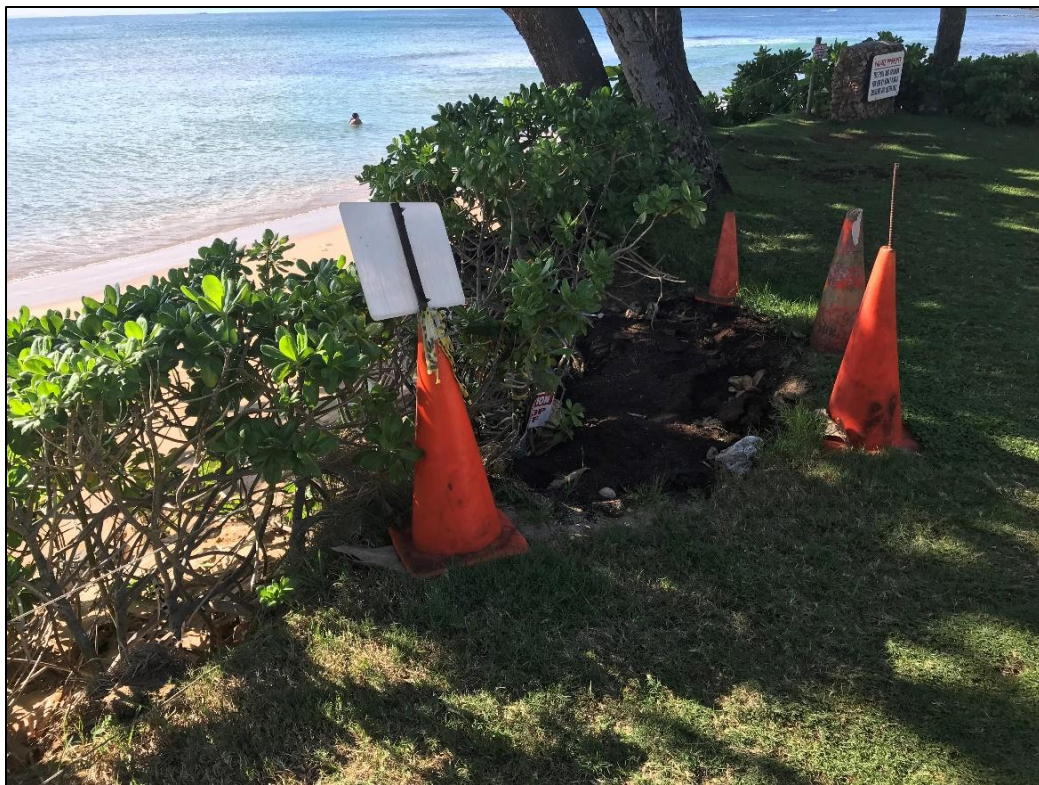
Figure 4-13 Evidence of active erosion
