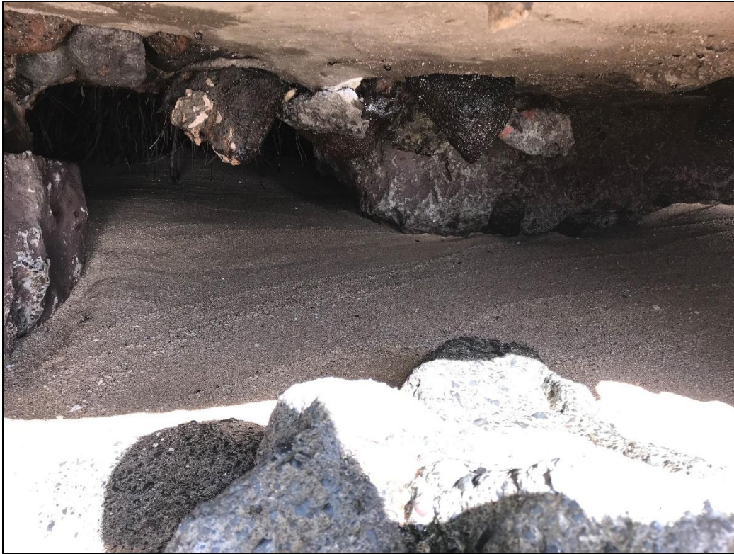
Figure 4-8 Void under seawall due to undermining
