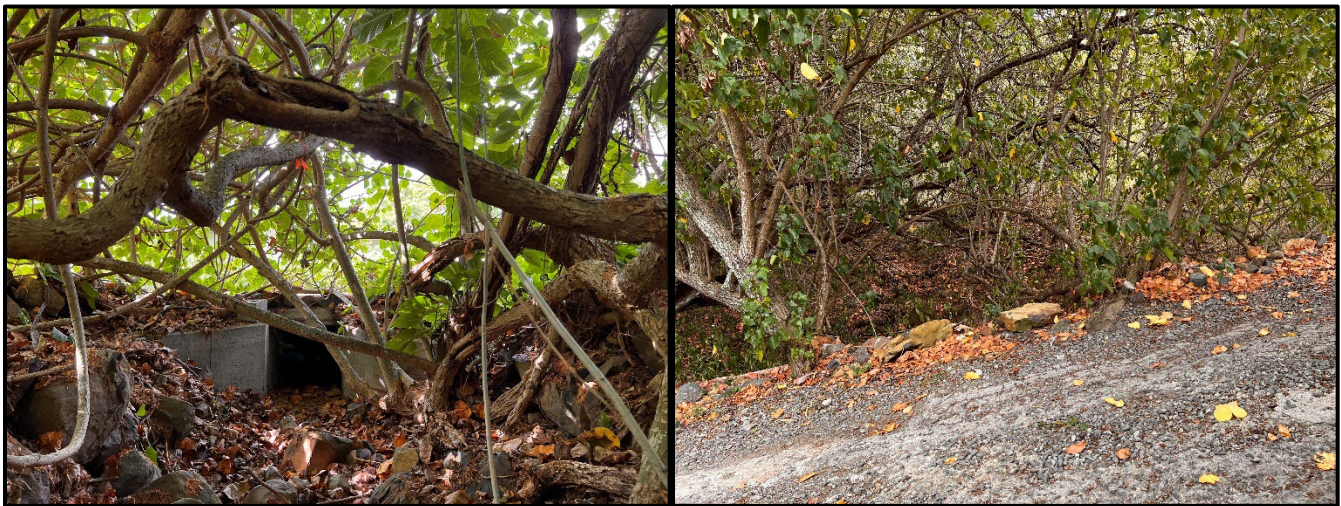
Figure 11. Storm Drain (left) and Intermittent Streambed (right) Located on Conservation Parcel adjacent to Existing, Non-Compliant driveway and within Road & Utility Easement (source: Don King)
