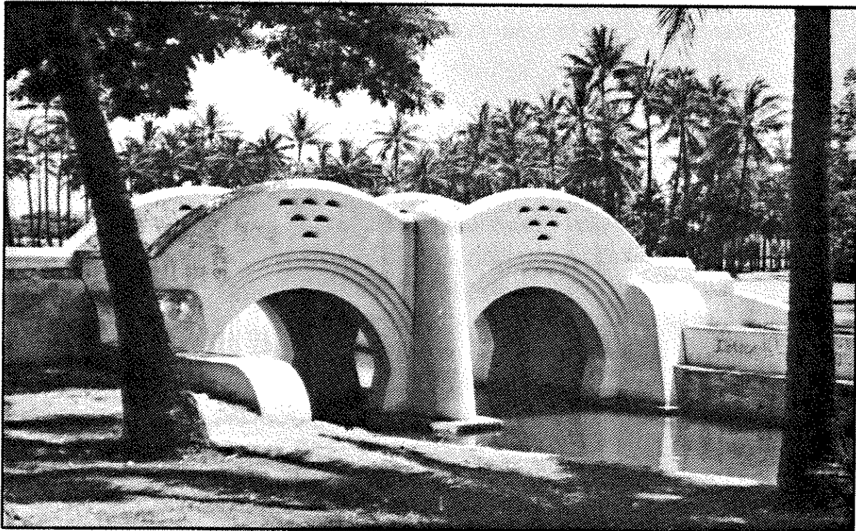
Plate 10 Concrete arch bridge at the outlet of the canal into the first lagoon. This bridge will be retained.
