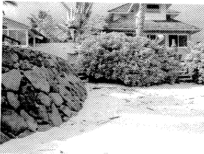
View of Parcel 11 seaward frontage. Seawall is hidden by naupaka vegetation. Curved seawall on left fronts Parcel 10.
