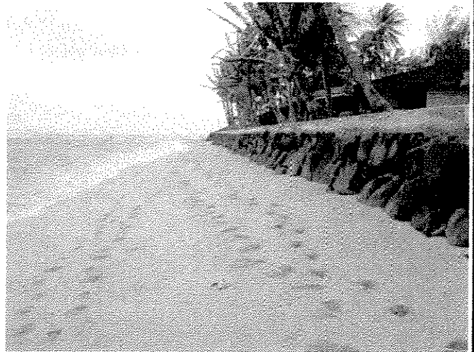
View eastward along the beach fronting the Mokuleia Beach Colony seawall. Note the narrow and steep beach profile.
