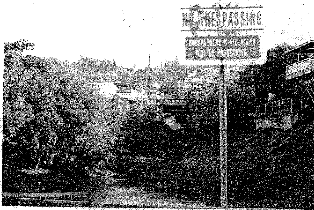
Top: Looking upstream from within stream at lower edge of box culvert beneath Naio St. bridge. Note undermining and erosion beneath culvert bed, and lack of cut-off wall which contributes to erosion.
