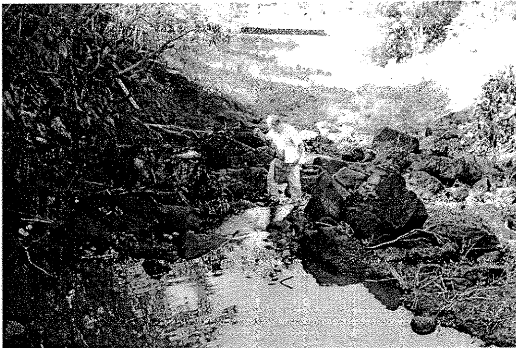
Top: Looking upstream from beneath Naio St. bridge at the existing upstream box culvert.
