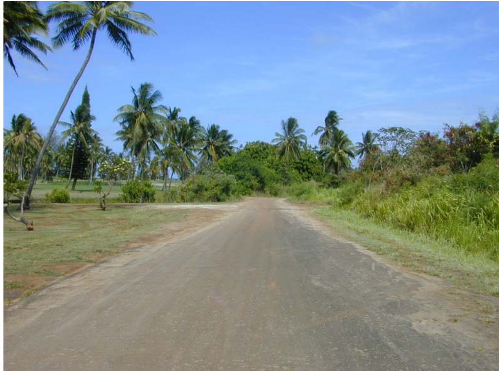
Figure 21a – Photo of un-named cane haul road extending to the Marine Camp site
