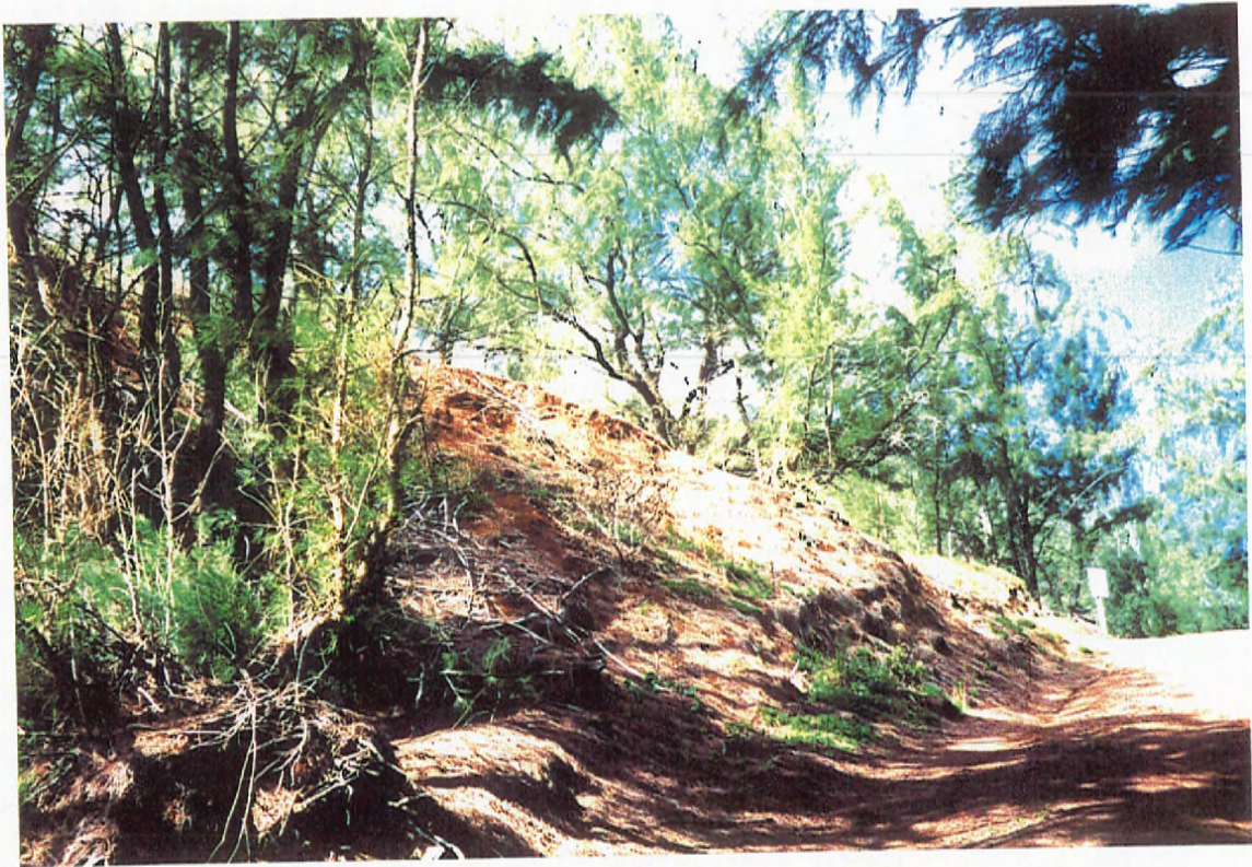
#11 and #12 Erosion under Ironwood trees causes tree failures
