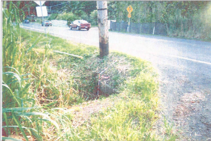
Figure 60. Photograph looking southwest at the culvert under Kamehameha Highway where the 'auwai (SIHP # 50-80-10-6758) begins in the project area.
