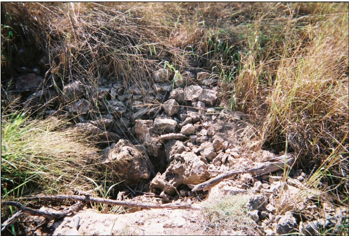
Figure 7. Rubble filled sinkhole (3 m diameter).
