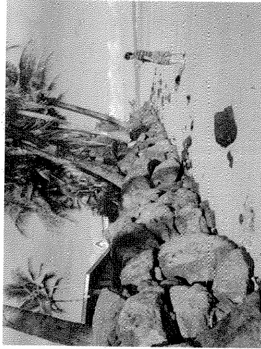
Existing condition of rebuilt shore protection structure. Photo date 12/28/04. Tide approx. +0.4 feet MLW.
