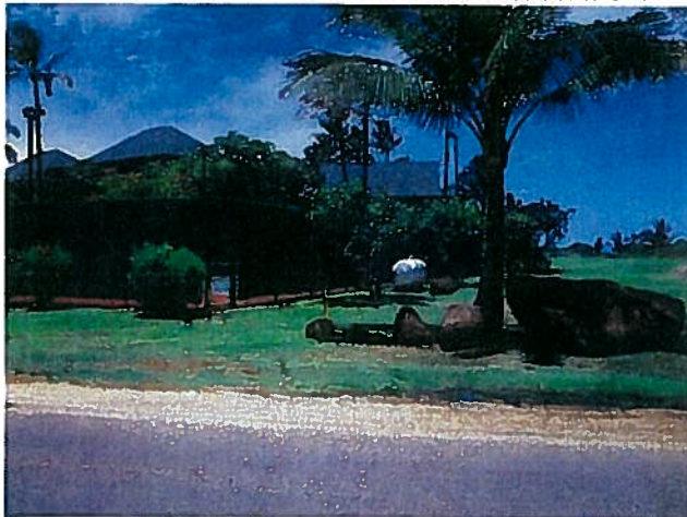
Photo 9: Aboveground propane AST observed at the Kaha Lani Resort.
