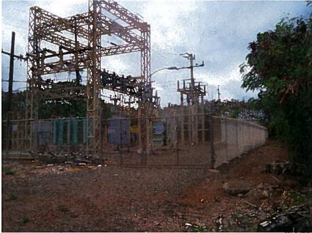
Photo 7: Kauai Island Utility Cooperative electric substation on an adjacent property.
