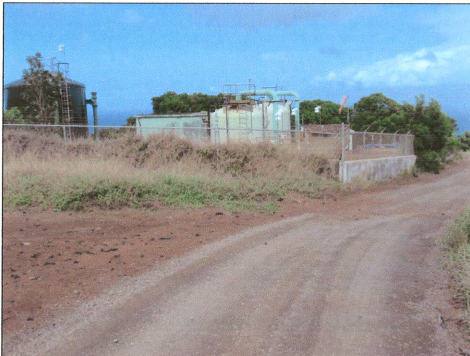
Photograph 2: View to the southwest along the existing access road for DWS facility.
