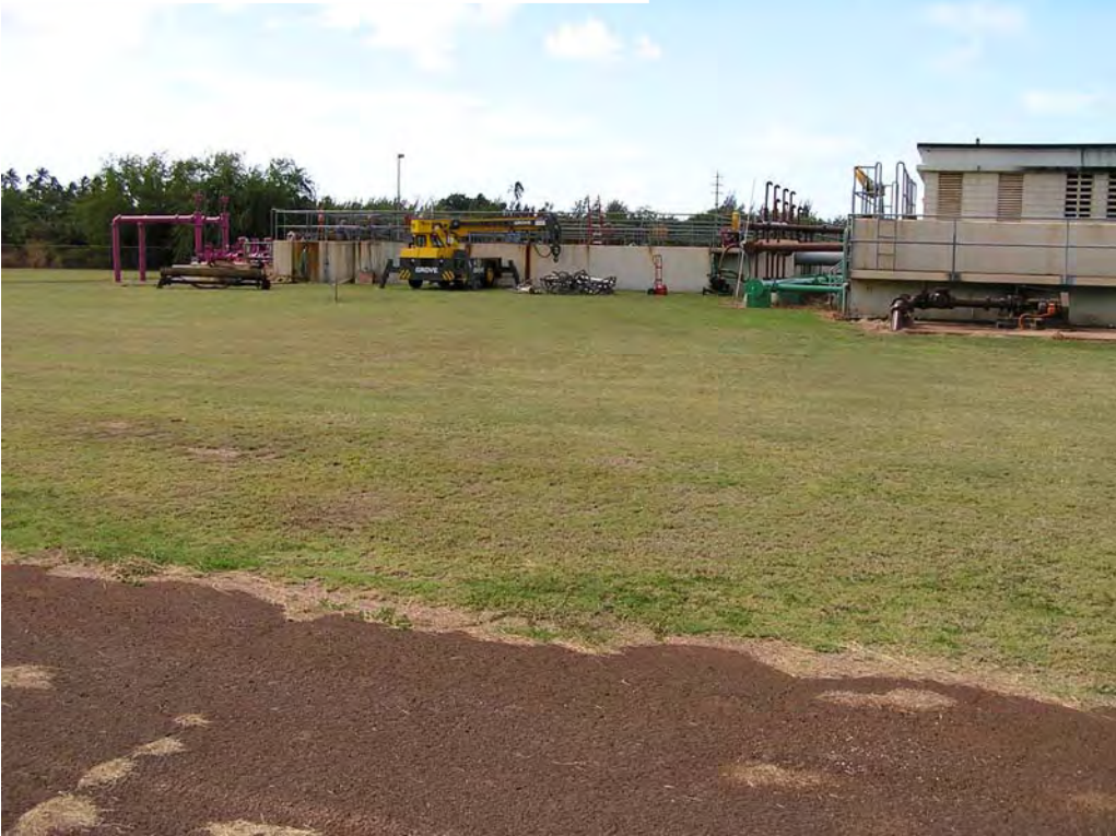
Figure 2. Existing Waimea WWTP. New structures for wastewater process to be placed here.
