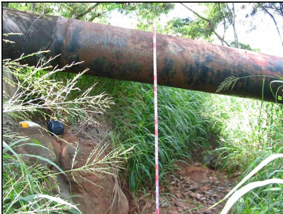
Figure 24. West view of 20-inch iron pipe crossing streambed at the base of Kalo'i Gulch
