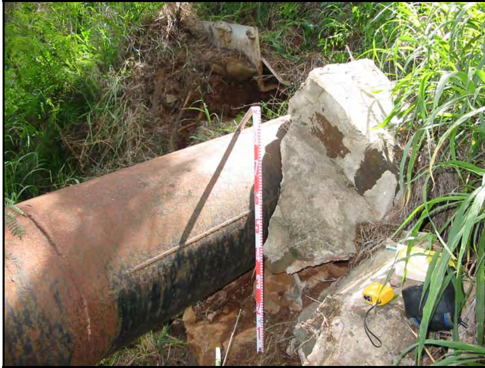
Figure 23. Southern end of 20-inch pipe, where a pre-fabricated ditch faces the iron pipe.
