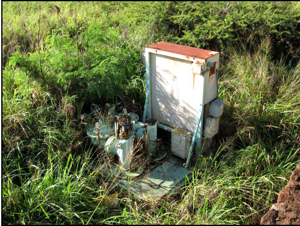
Figure 9. Southwest view of irrigation and control box in south-central portion of project area
