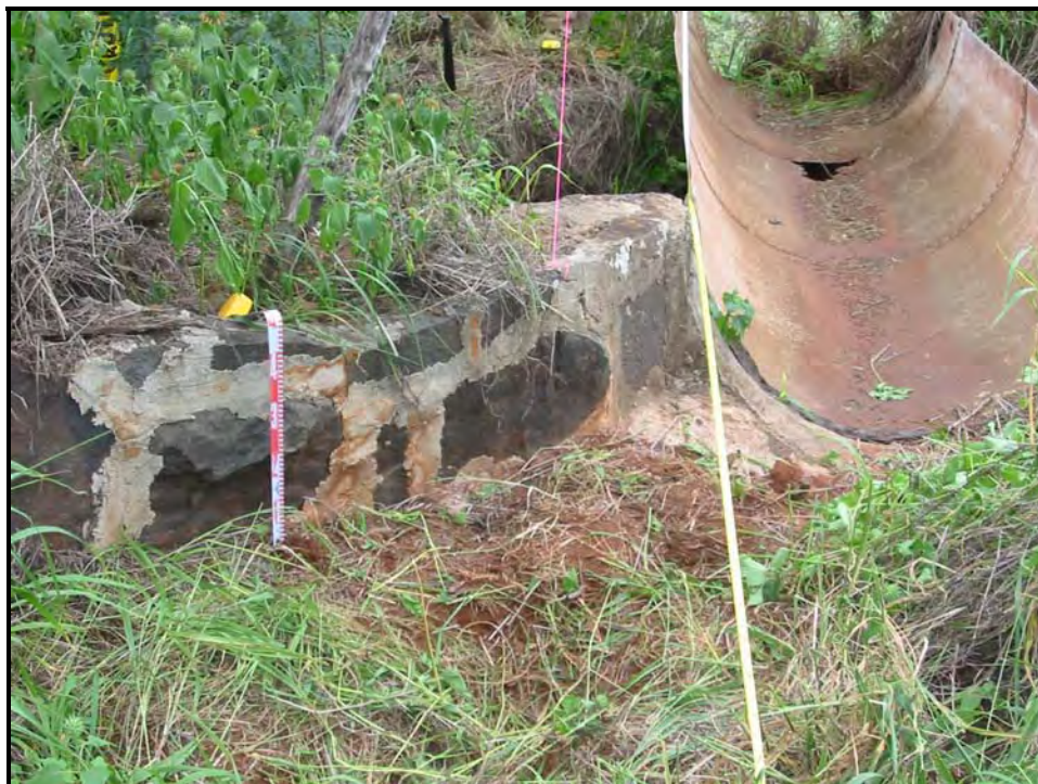
Figure 39. North view of landing area and cut basalt stone and mortar retaining wall
