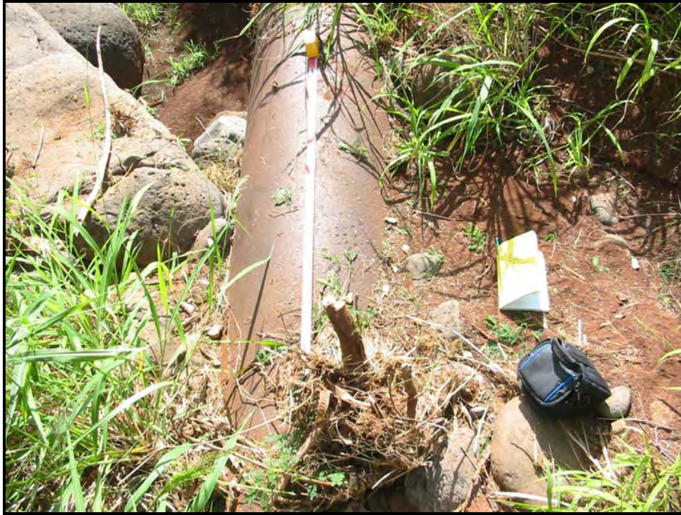
Figure 25. South view of northernmost section of iron pipe, where pipe goes underground
