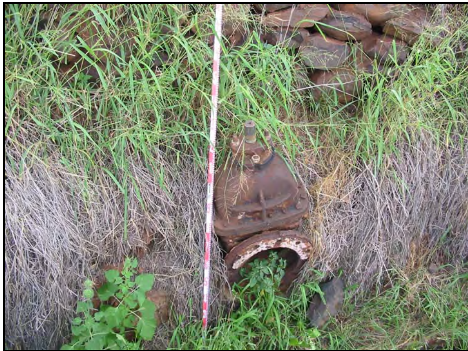
Figure 34. Valve observed as part of Site -6951
