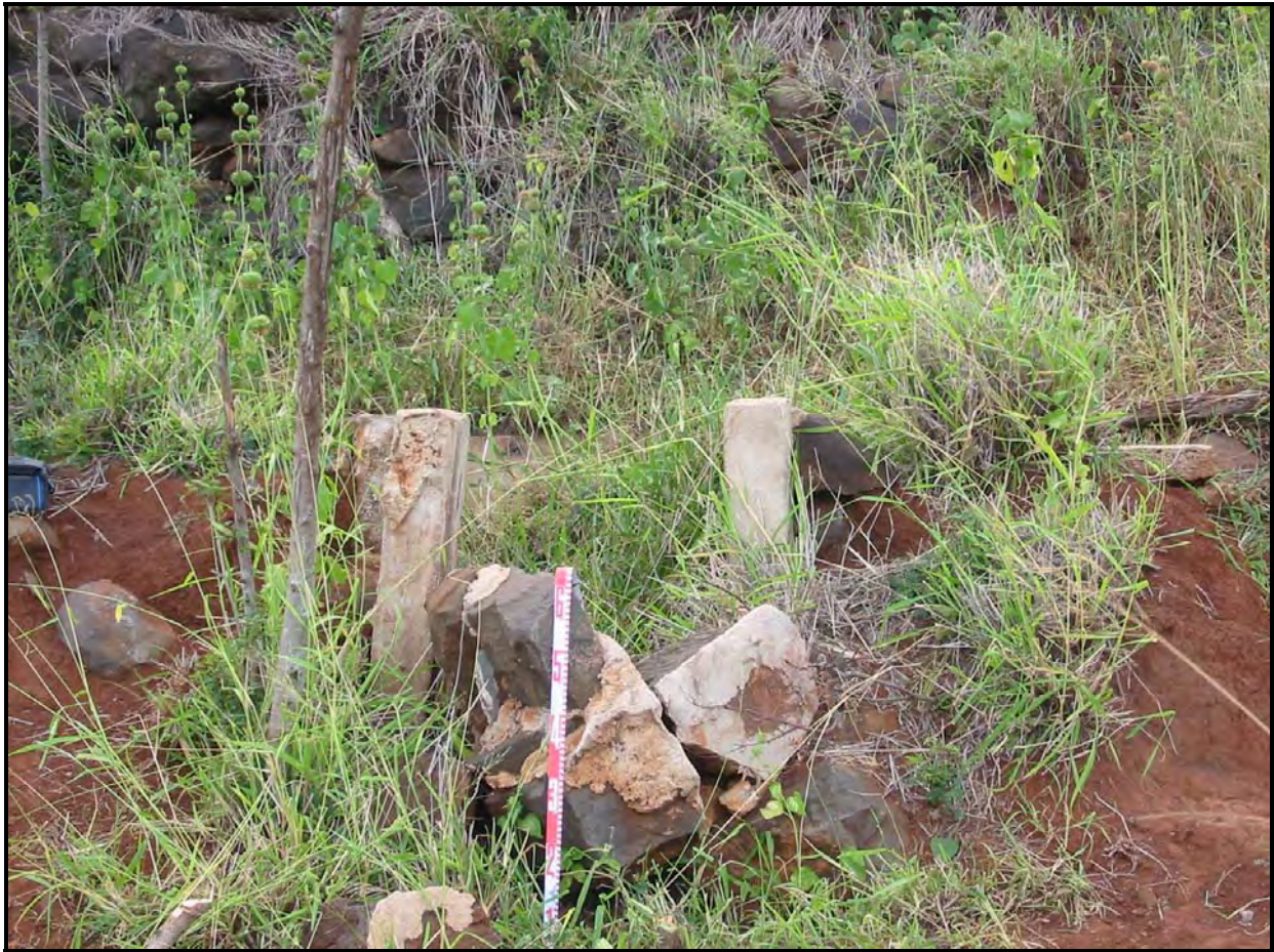
Figure 37. West view of collapsed outflow ditch, south of central outflow ditch and gate
