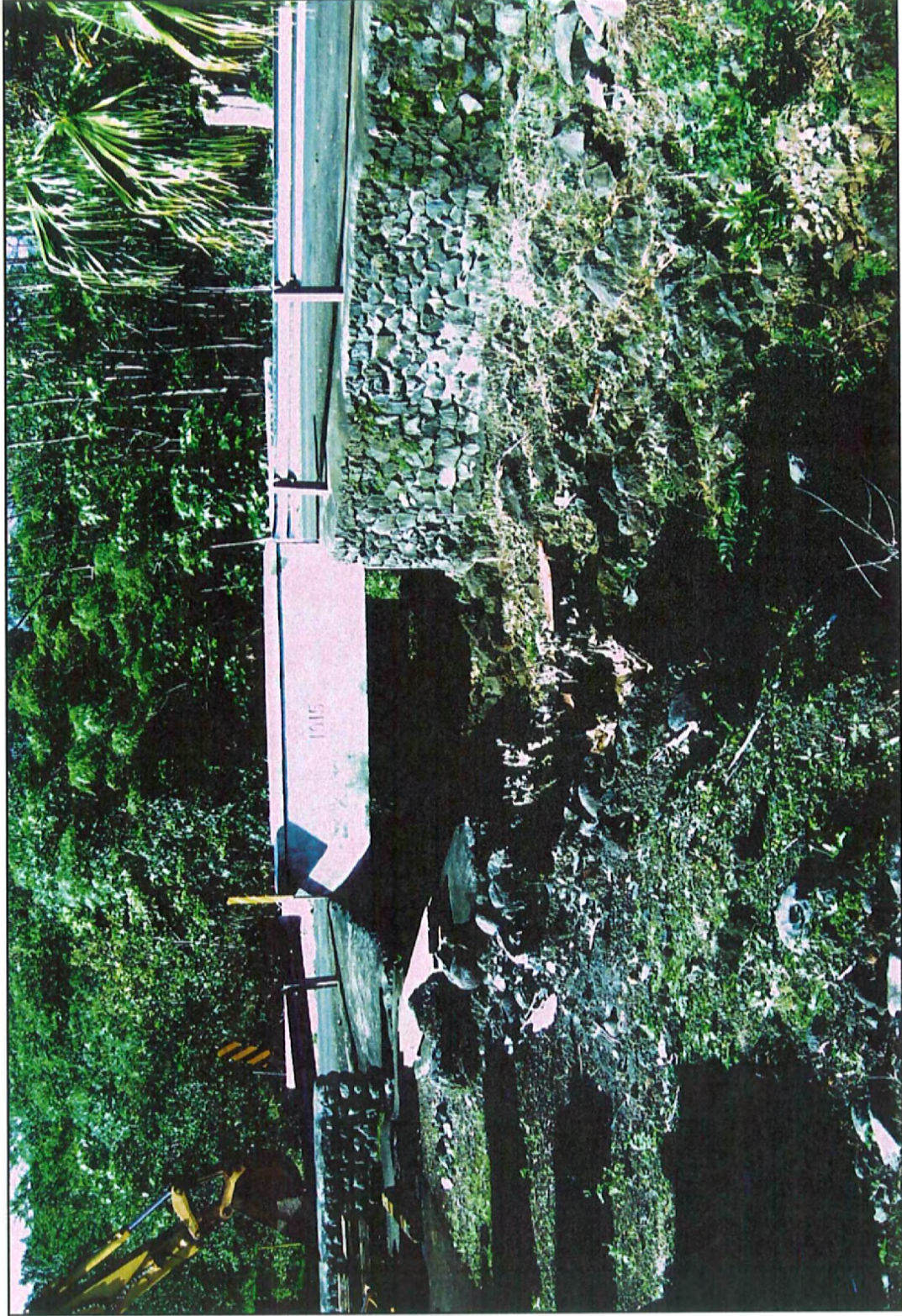
Figure 4: View West of Bridge and Culvert (SIHP No. 50-50-06-1636 Features A and B)
