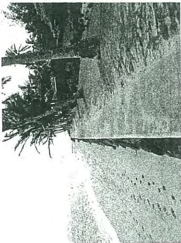
View eastward along the top of the seawall fronting the Mokuleia Beach Colony. Note the narrow beach.
