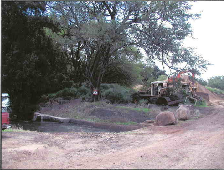
Photograph 1: View to the southeast across intake in left foreground. Project area southeast of equipment.
