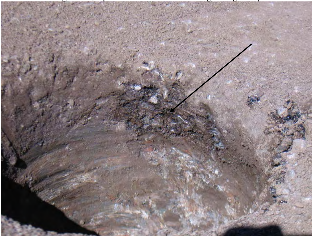
Photo 13A--- Water flowing through pavement layer cracking
