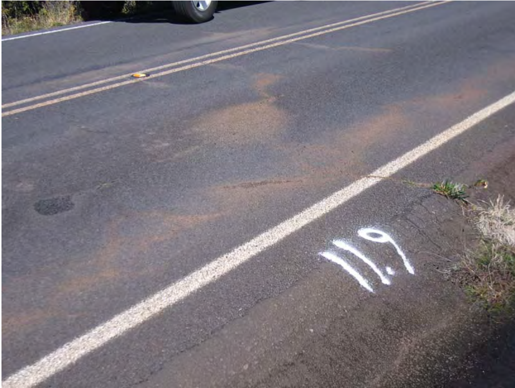
Photo #4---Segment 2 MP 11.9, Typical pavement distress, note water in paved water way
