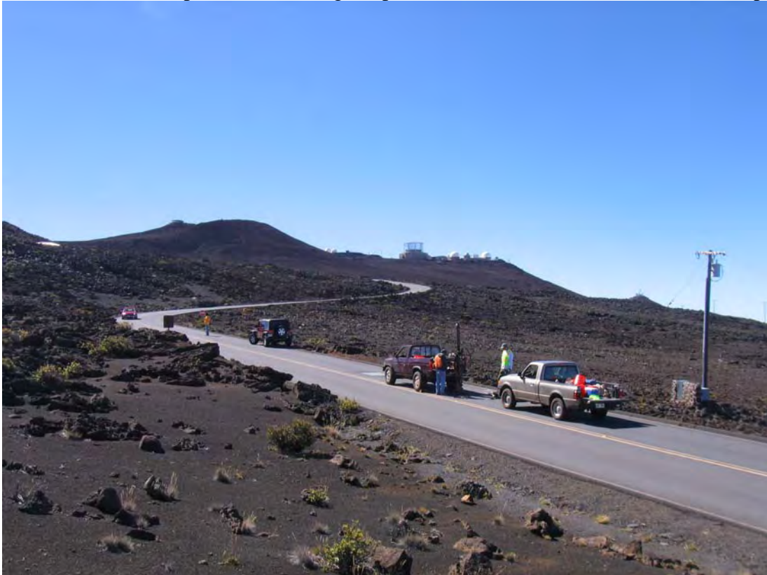
Photo #10 ---Segment 4, Auguring at MP 20.3, Note: Start of Utility line in Rdwy.
