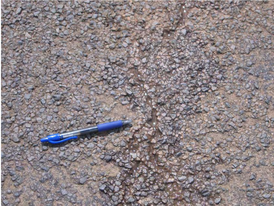
Photo #9 ---Close-up of water in fatigued pavement, note fine on the surface of the pvt.
