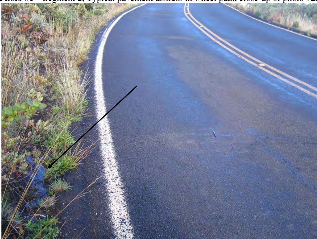
Photo #2 ---Segment 2, Pavement distress adjacent to water in the roadway ditch line
