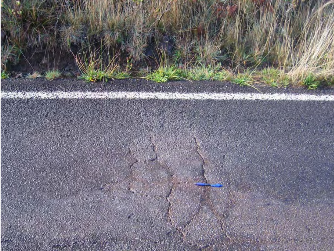
Photo #1 ---Segment 2, Typical pavement distress in wheel path, close-up of photo #2.
