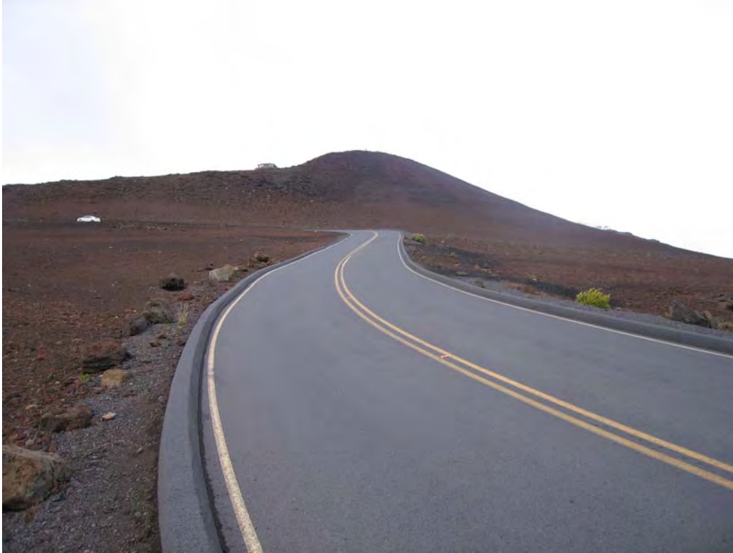
Photo #22 -----Section 4, newer roadway surface. Not yet chipped with low to moderate transverse and longitudinal cracking.
