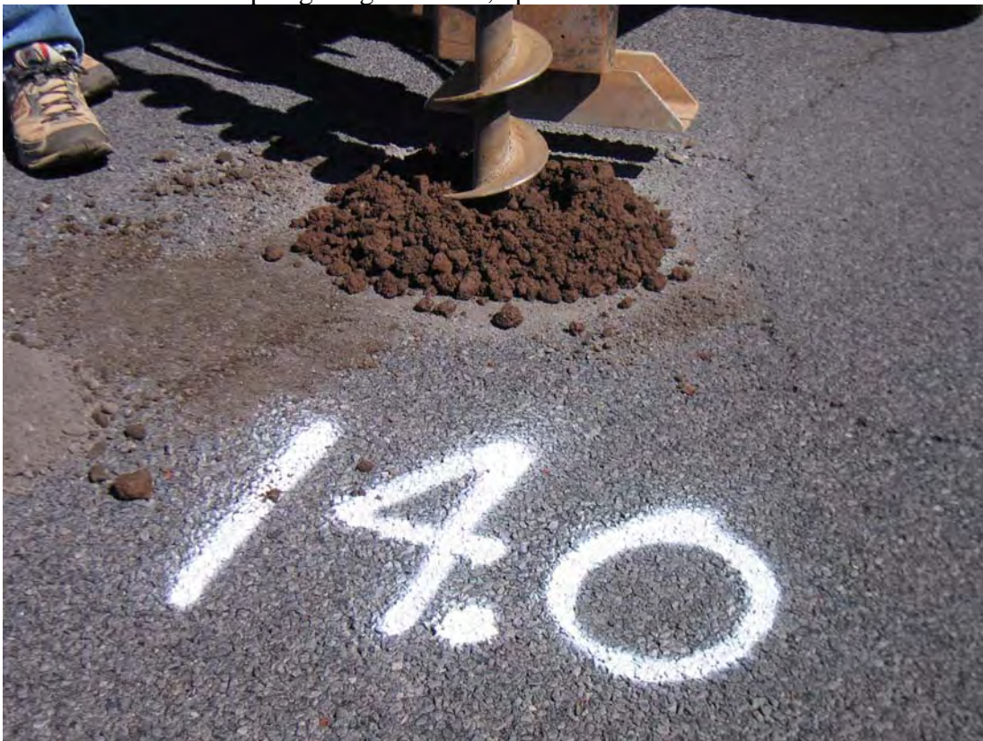
Photo #12---Very wet subgrade material at MP-14
