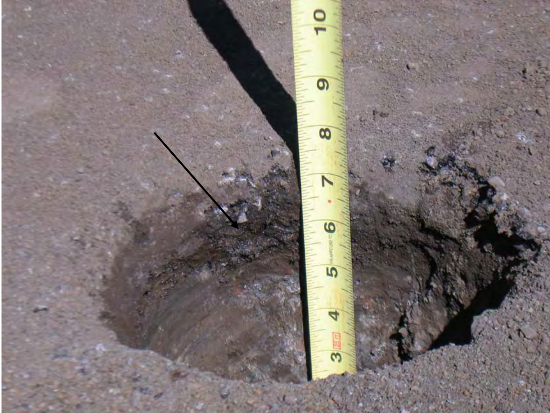
Photo #13--- Auger hole, Uphill lane- note water flowing through the pavement.
