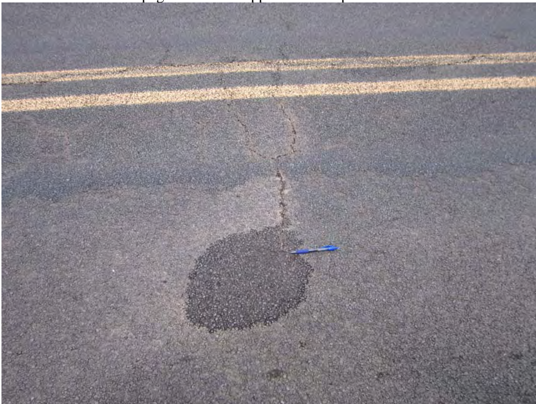
Photo #8 ---Section 2, Water seepage from fatigued roadway section
