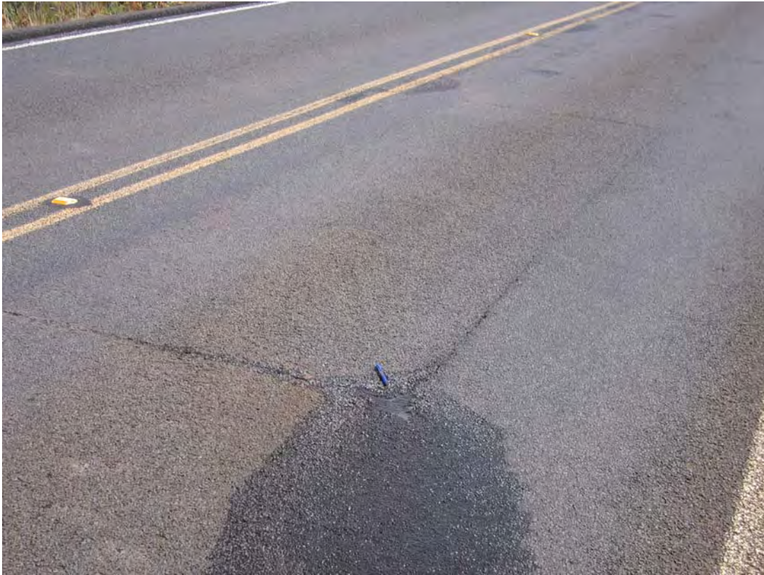
Photo #7 ---Water seepage from what appears to be a patched area in Section 1
