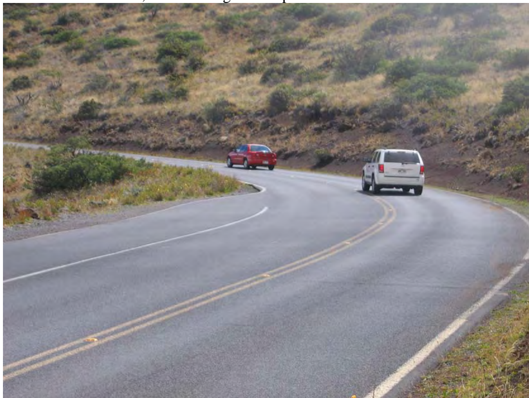
Photo #21 ----Section 3, low to moderate transverse and longitudinal cracking
