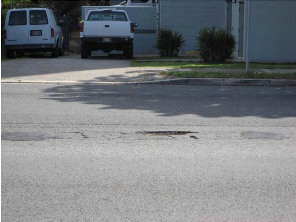
Photo P-81: Pensacola Street Pothole
