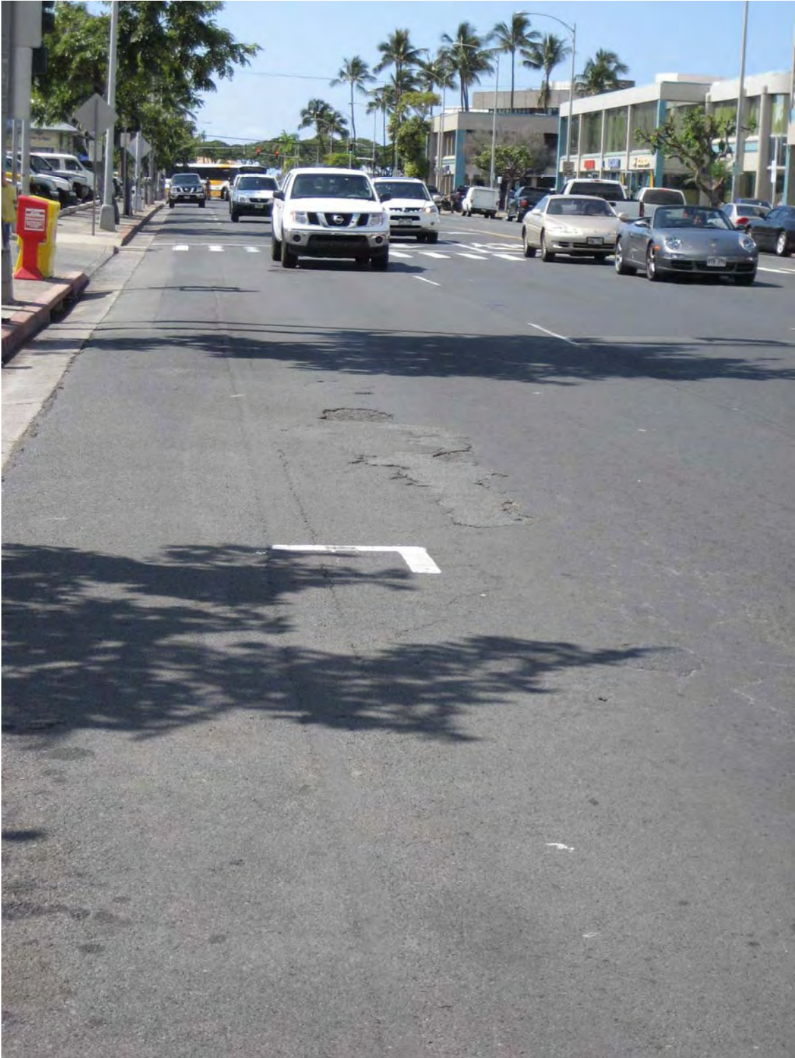
Photo P-67: Ward Avenue Pothole & Deteriorating Patching
