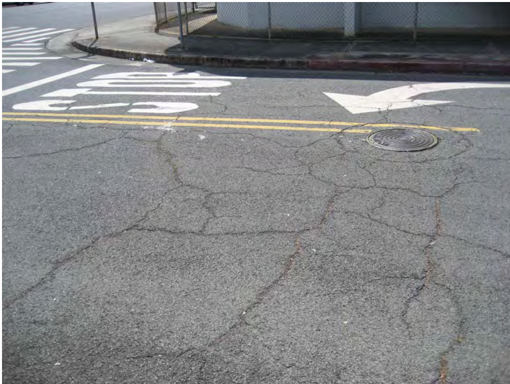
Photo P-104: Hoolai Street at Piikoi Street Block Cracking
