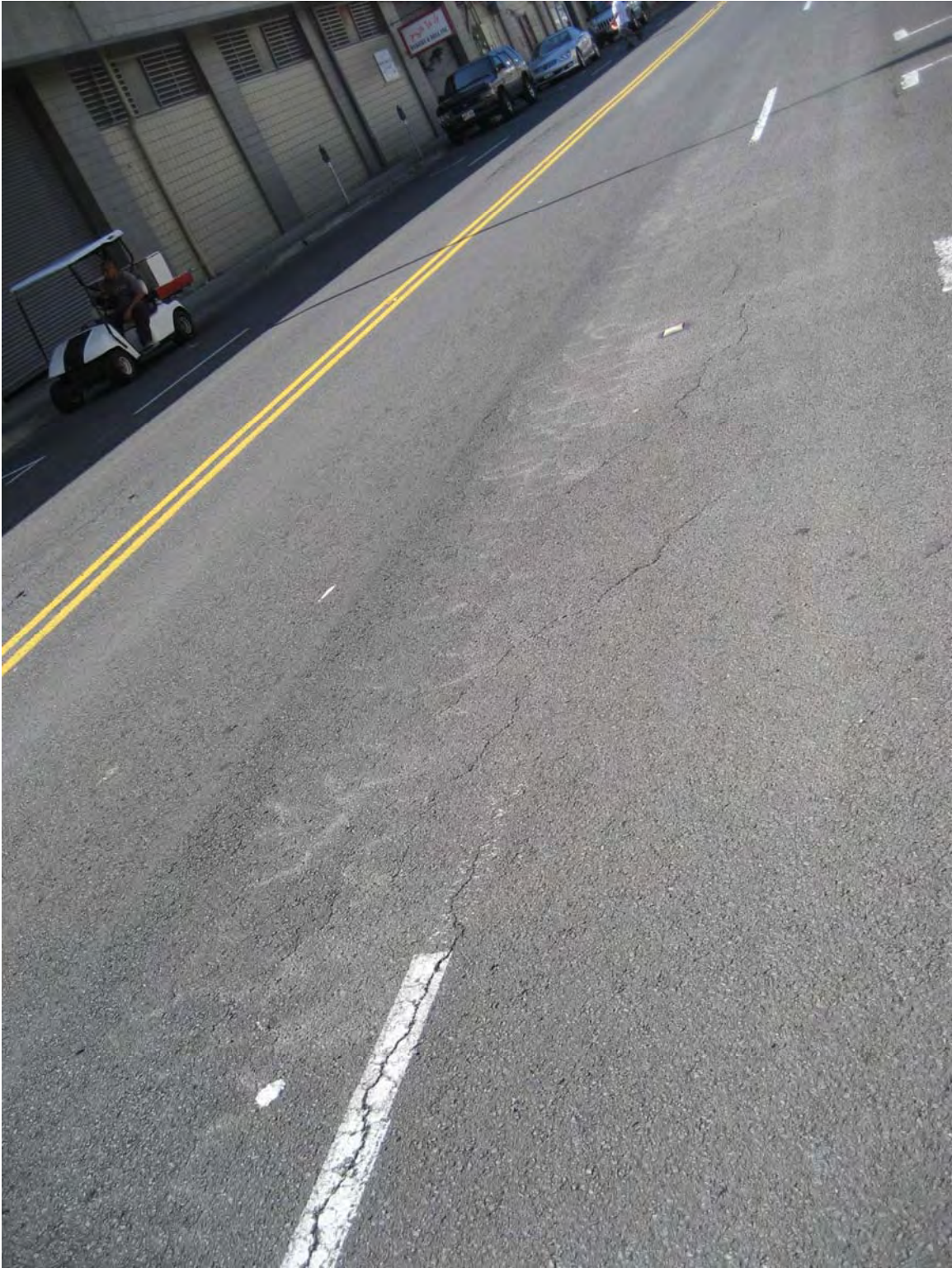
Photo P-13: Cooke Street Rutting
