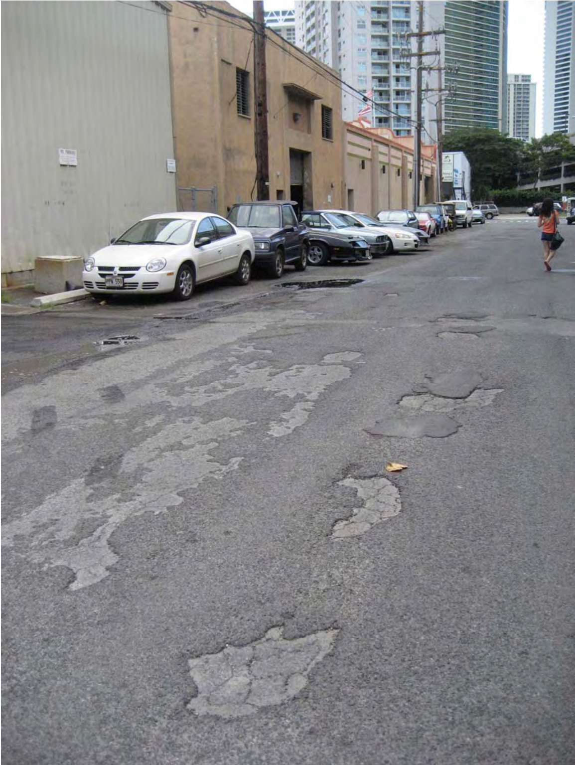
Photo P-163: Kawaiahao Street Rutting & Deteriorating Patching
