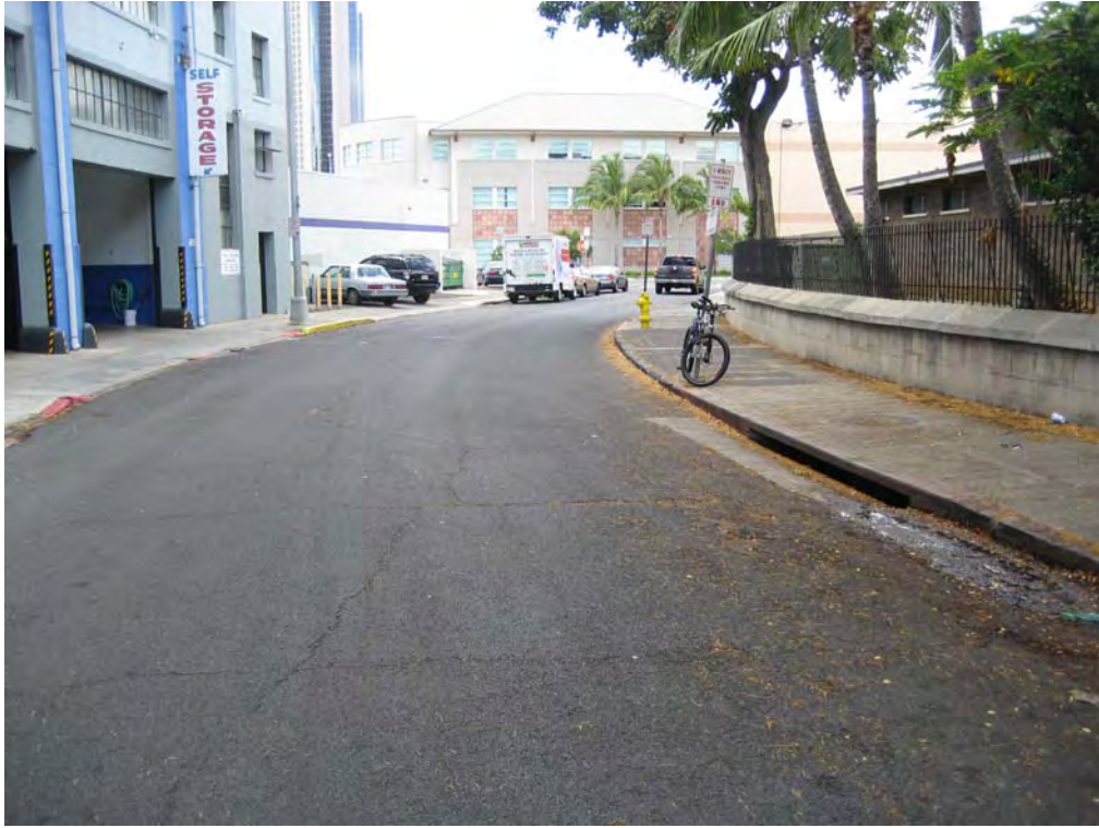
Photo P-192: Mission Lane Block Cracking
