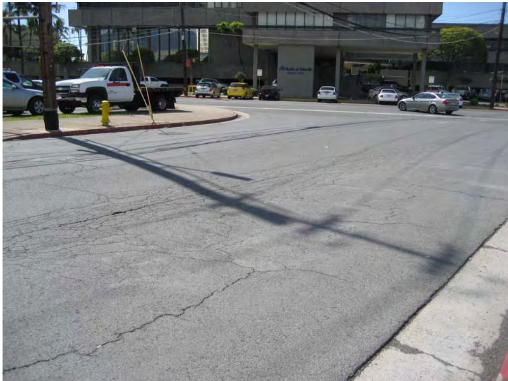
Photo P-58: Kamani Street Alligator & Block Cracking
