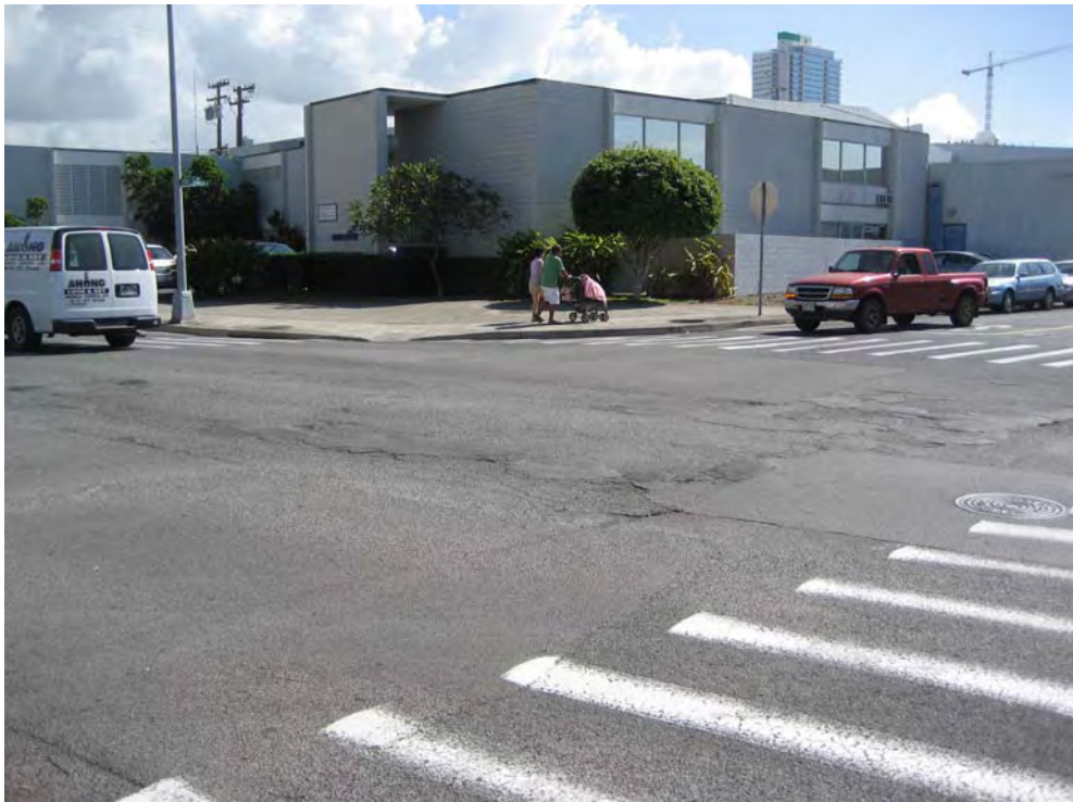
Photo P-10: Cooke Street at Halekauwila Street Raveling & Block Cracking
