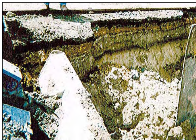
Figure 46. Kaka'ako Improvement District 7 (ID-7), southeast profile near Kamake'e and Auahi Street showing thin dark "A" horizon below street fill gravel, crushed coral layers and above calcareous sand, (Souza et al. 2002)
