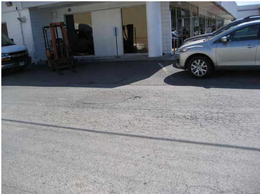
Photo P-26: Koula Street Alligator Cracking
