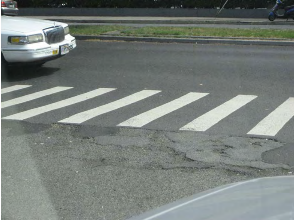
Photo P-111: Hopaka Street at Piikoi Street Raveling & Deteriorating Patching
