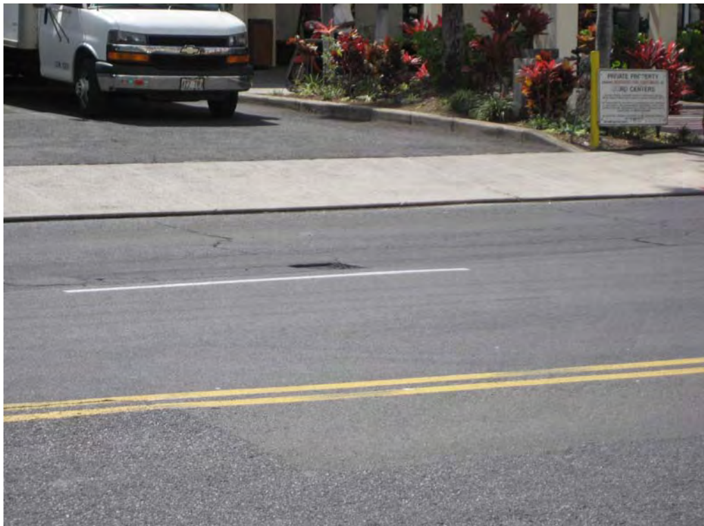
Photo P-129: Auahi Street Pothole
