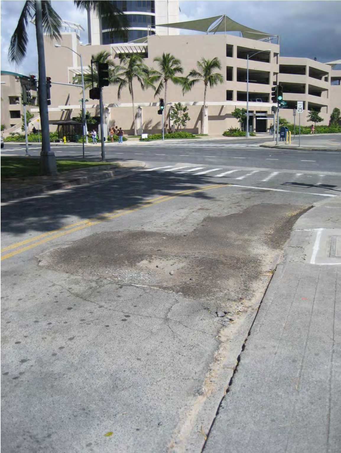
Photo P-42: Coral Street Deteriorating Patching
