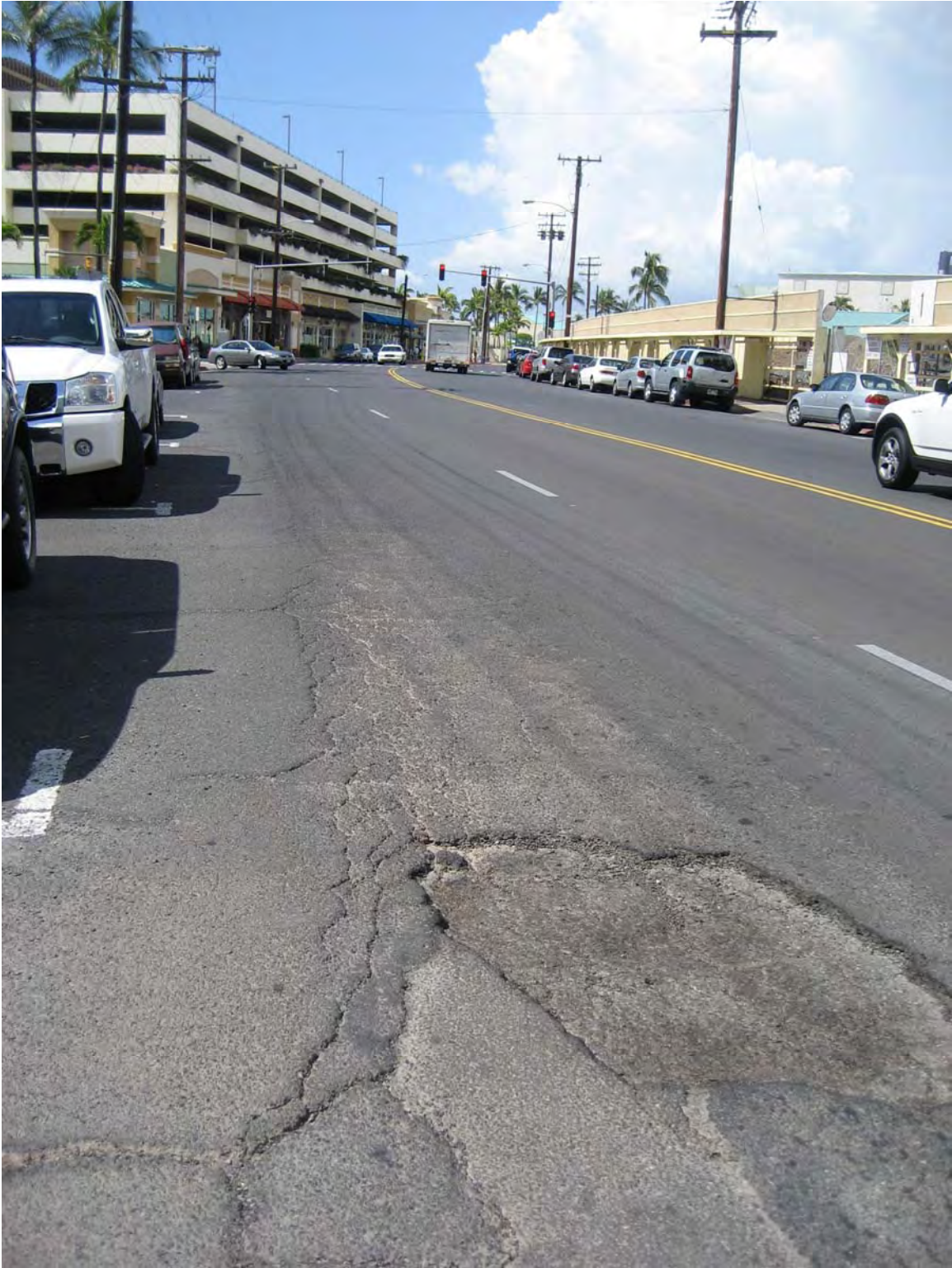
Photo P-132: Auahi Street Pothole
