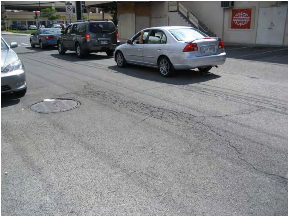
Photo P-113: Kona Street Alligator & Block Cracking & Raveling
