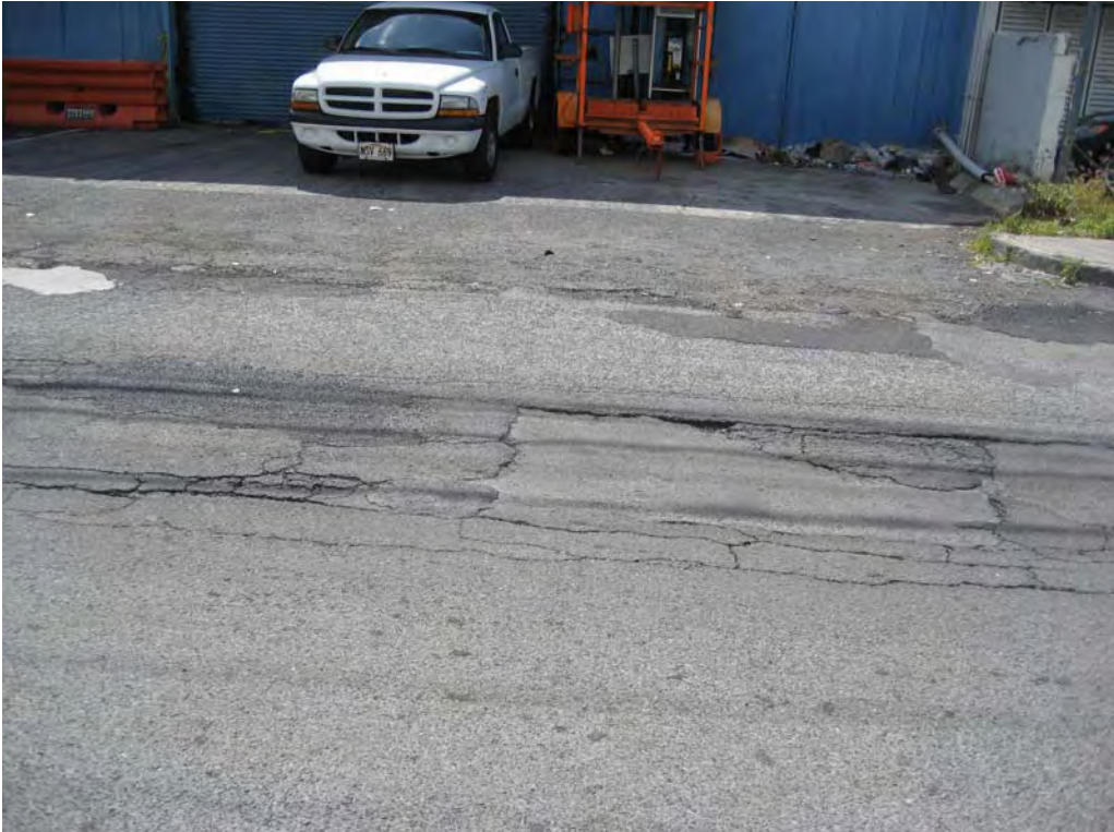
Photo P-117: Kona Street Block & Longitudinal Cracking
