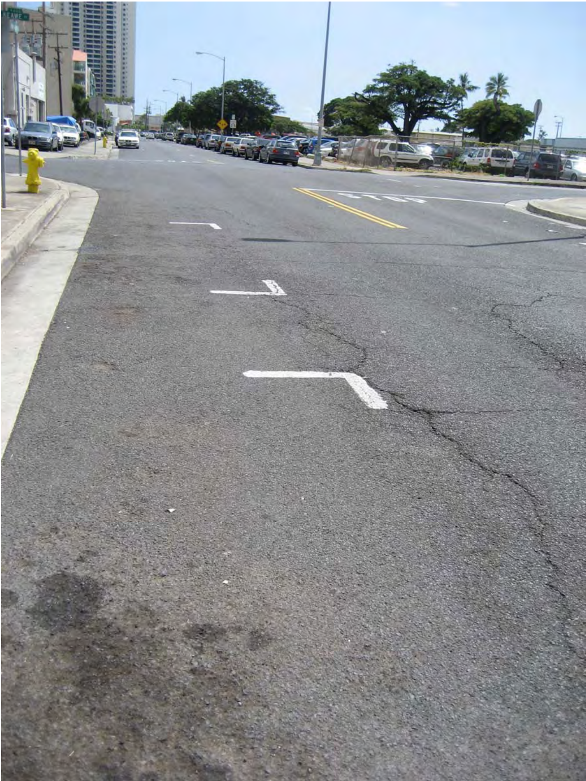
Photo P-147: Pohukaina Street Longitudinal Cracking
