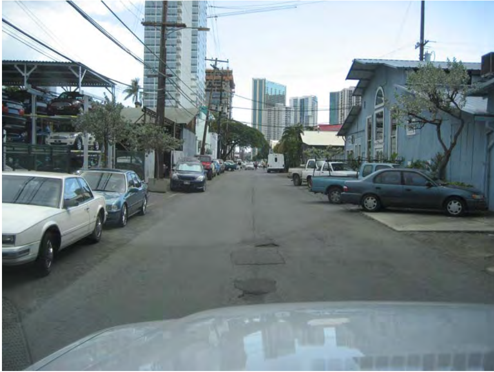
Photo P-181: Waimanu Street Potholes, Deteriorating Patching & Longitudinal Cracking
