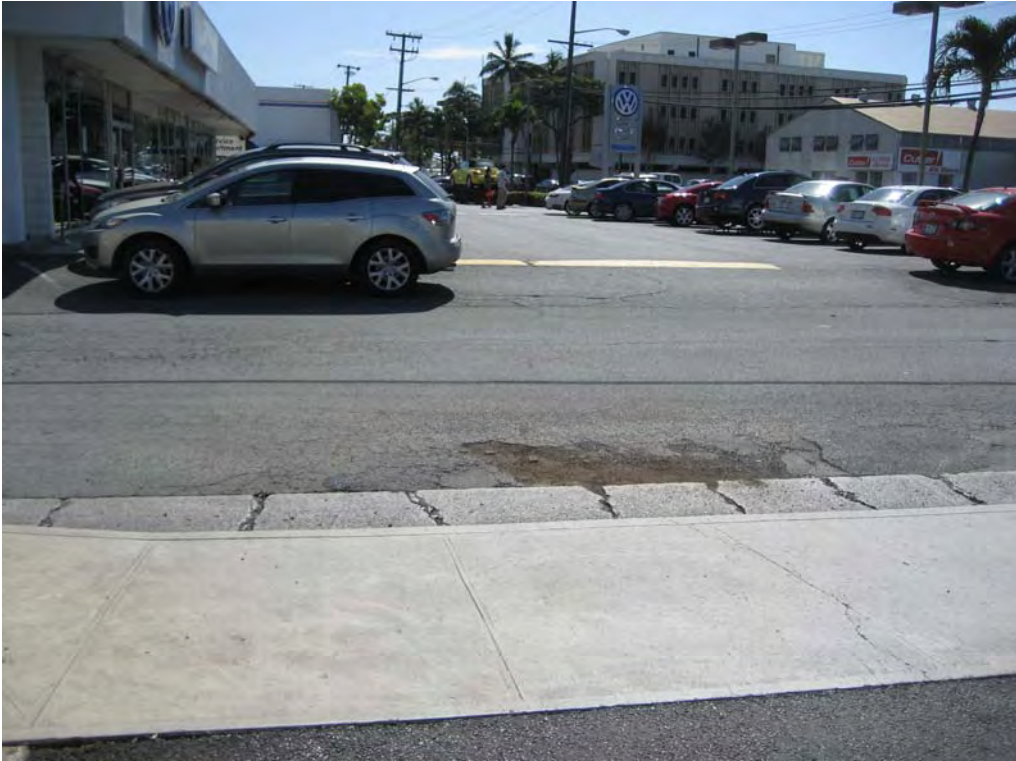
Photo P-25: Koula Street Pothole & Alligator Cracking
