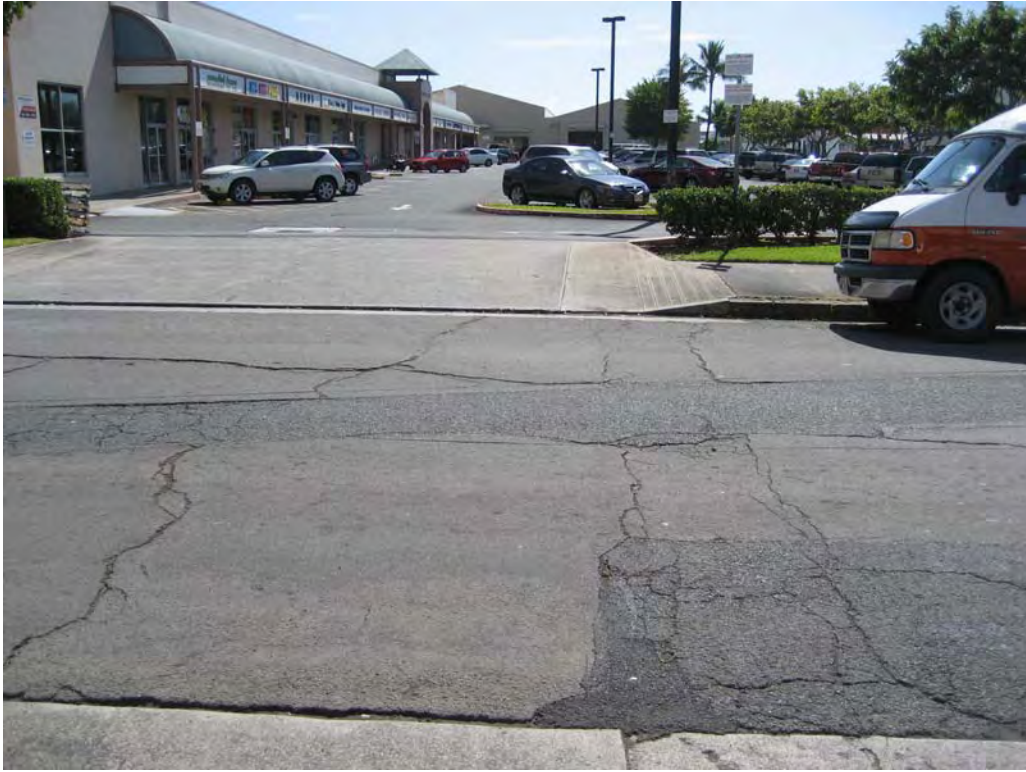
Photo P-37: Keawe Street Block Cracking
