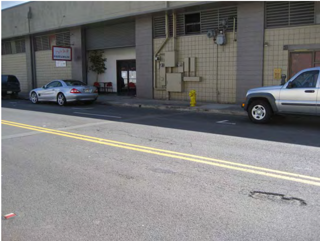
Photo P-17: Cooke Street Pothole
