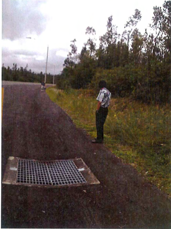
Grated Inlet Drywell in County ROW fronting the Proposed Site on Mohouli Street (10/18/07)
