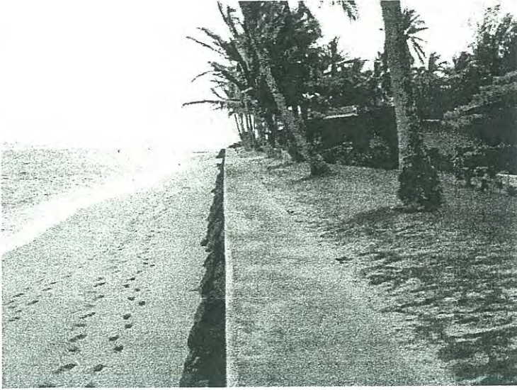
View eastward along the top of the seawall fronting the Mokuleia Beach Colony. Note the narrow beach.
