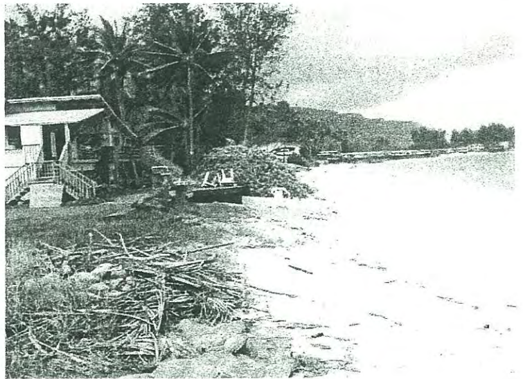
Shoreline fronting Parcel 20 on east side of stream. Note debris line at edge of vegetation.
